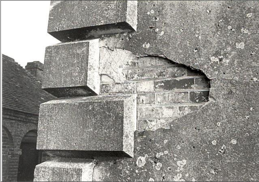
Stone quoins on the north-west corner. The scored joints of the brickwork show clearly, where the stucco has broken away.
