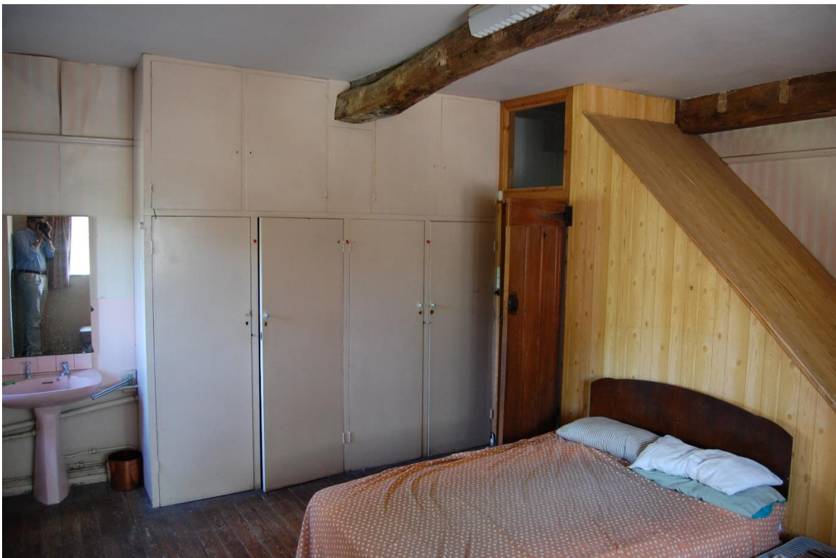
Examples of the crude late 20 th -century adaptations: as hoc partitions, corridors and washbasins.
