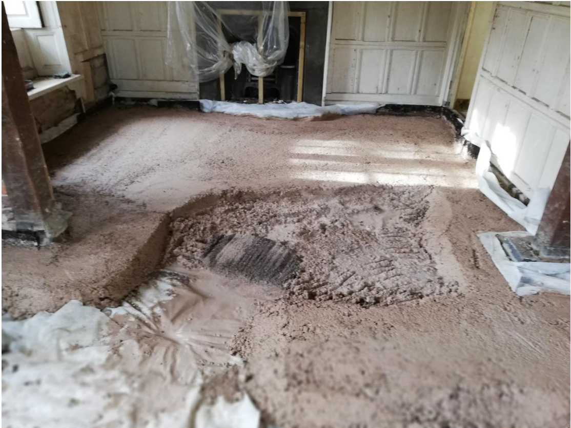
Floor slab construction underway in the sitting room. Lime-based screed is laid on wood wool board; oak floorboards fixed on battens were then laid on top.
