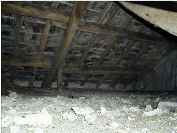
Inside the roof space above the hall chamber, before restoration. Note the plaster rising almost up to lower purlin height, showing that the ceiling was originally open to the rafters.
