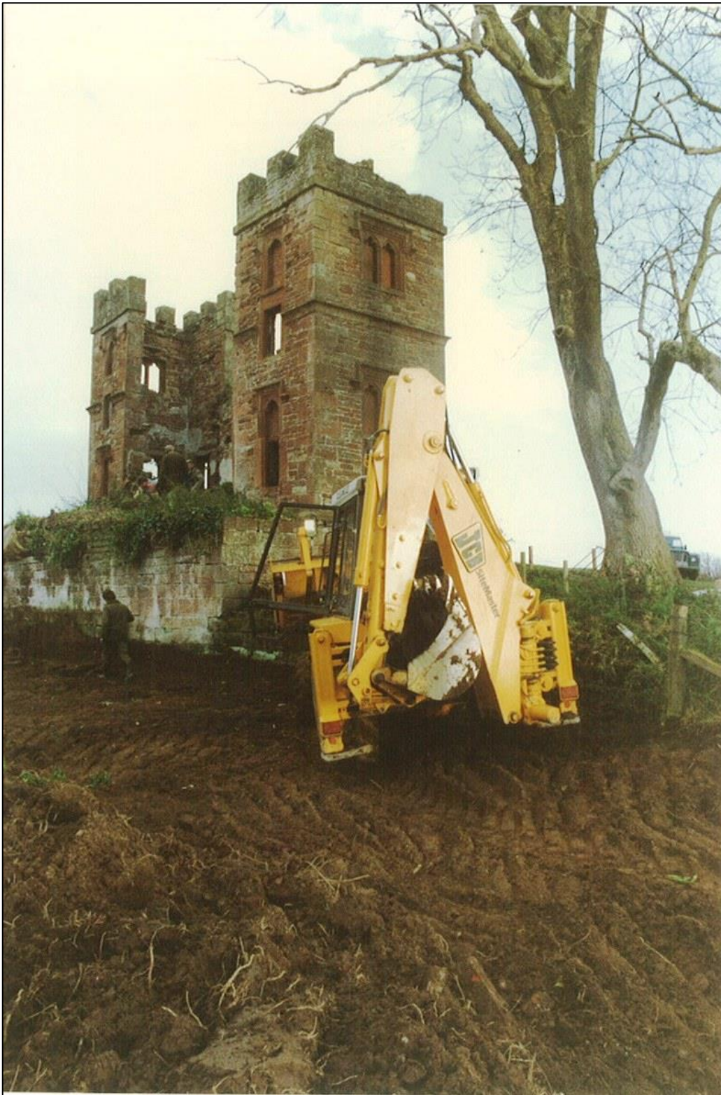
Clearing away soil in front of the terrace in 1989, to discover the state of the foundations – what this revealed was the platforms on which the coops could be fixed.
