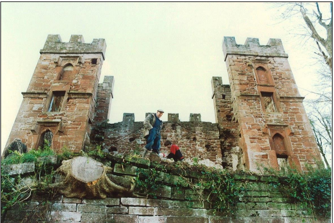
The front parapet as damaged by a tree stump.
