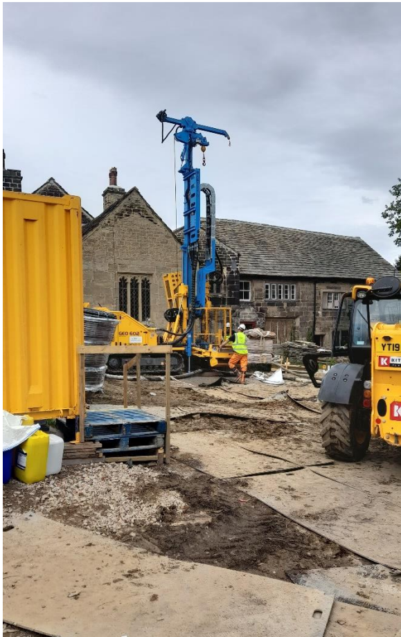
Drilling the bore holes for ground source heating. Six bore holes were drilled to a depth of 143 metres. The process proved easier than anticipated, to everyone's relief.
