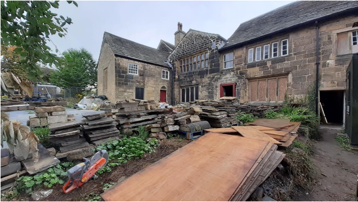
By summer 2022, the scaffolding was down and site set-up complete. The flagstones from the Great Hall had been recorded and were now carefully stacked while underfloor heating was installed.
