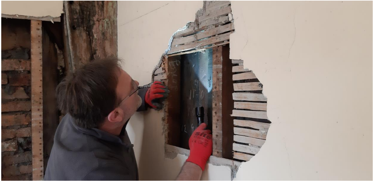
With traces of paint clearly apparent on the revealed corner jowl post, investigations were taken further.
