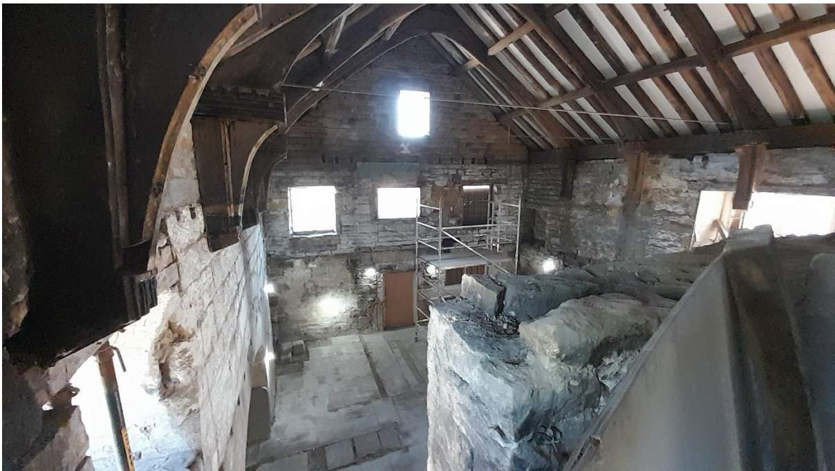
The removal of the cottage in the southeast end of the Great Hall allowed a first glimpse into the Great Hall from high level, a view that is now familiar as a key element in the conversion scheme.
