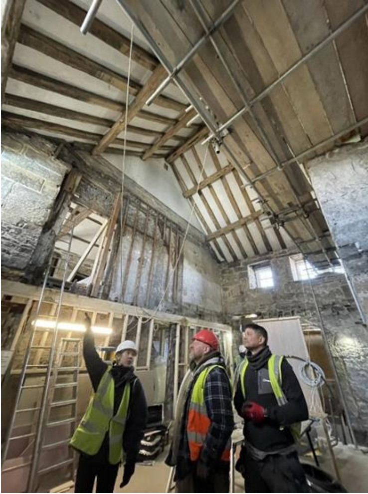
During the clearance of the cross passage, the original doorway into the first-floor hall was discovered in 1320s framing. Here, architect Karen Lim briefs Kevin Woods, plasterer (in the red hat) Michael Bloom, joiner
