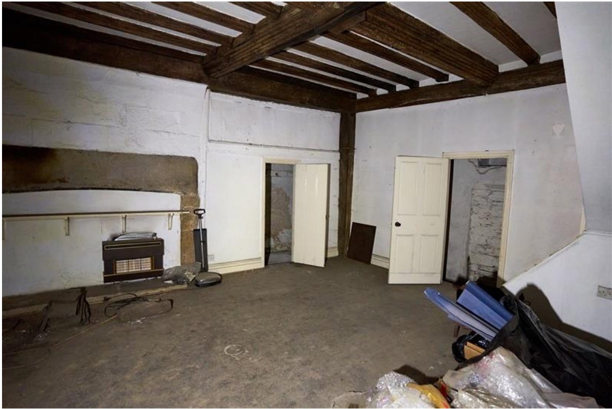
Top: the ground floor of the Parlour Block in 2020. The slope of an inserted cottage staircase is in the foreground. The blocked doorway to the Solar Block was a cupboard.
