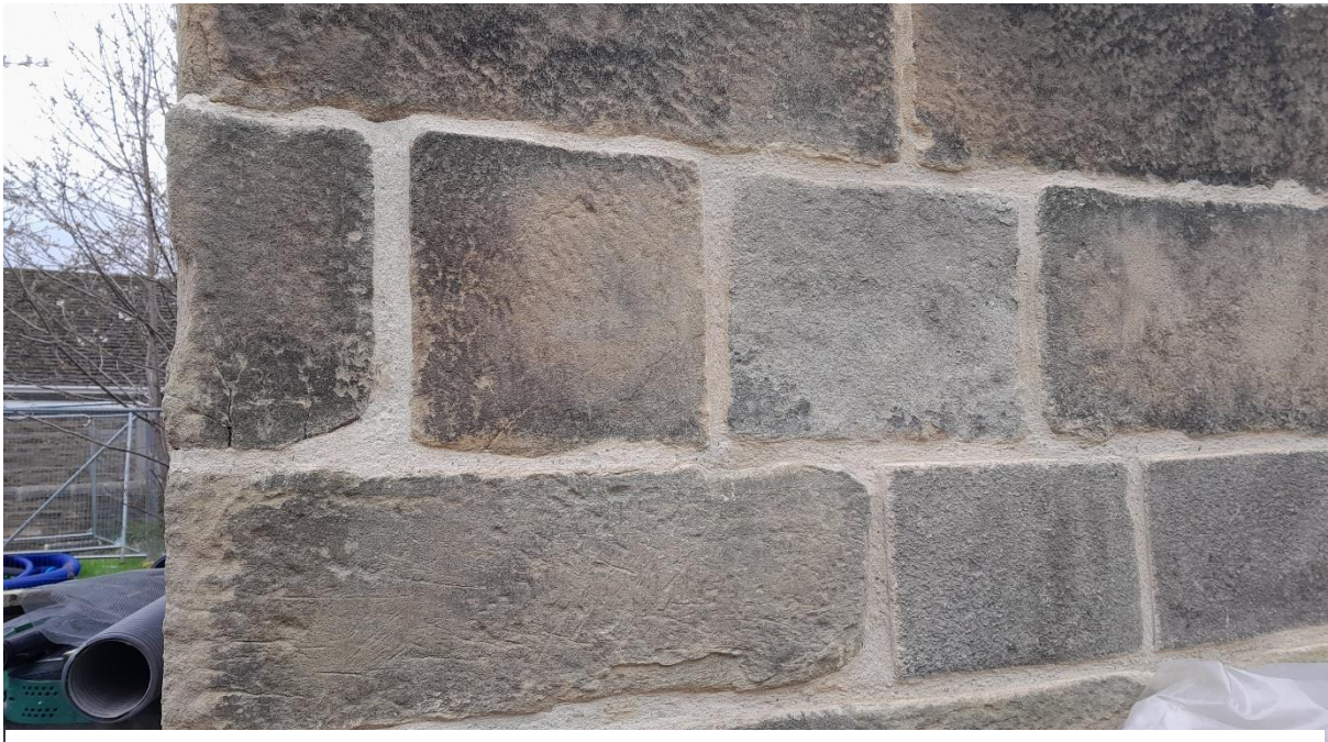
From top left: slaking lime on site; tile repairs in one of the many wall cavities, here in the partition wall of the Great Hall; a sample of external pointing, the mortar mix and style refined with great care by stone mason Kevin Woods and his team.
