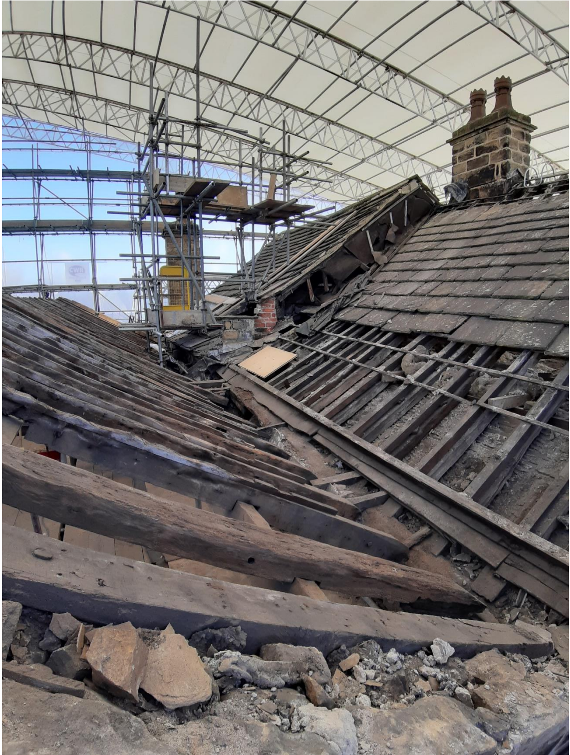
View southwest along the length of the Solar and Parlour Blocks during re-roofing, with the Chapel at the far end. While some rafter ends had rotted, the roof was not in as bad a condition as feared.
