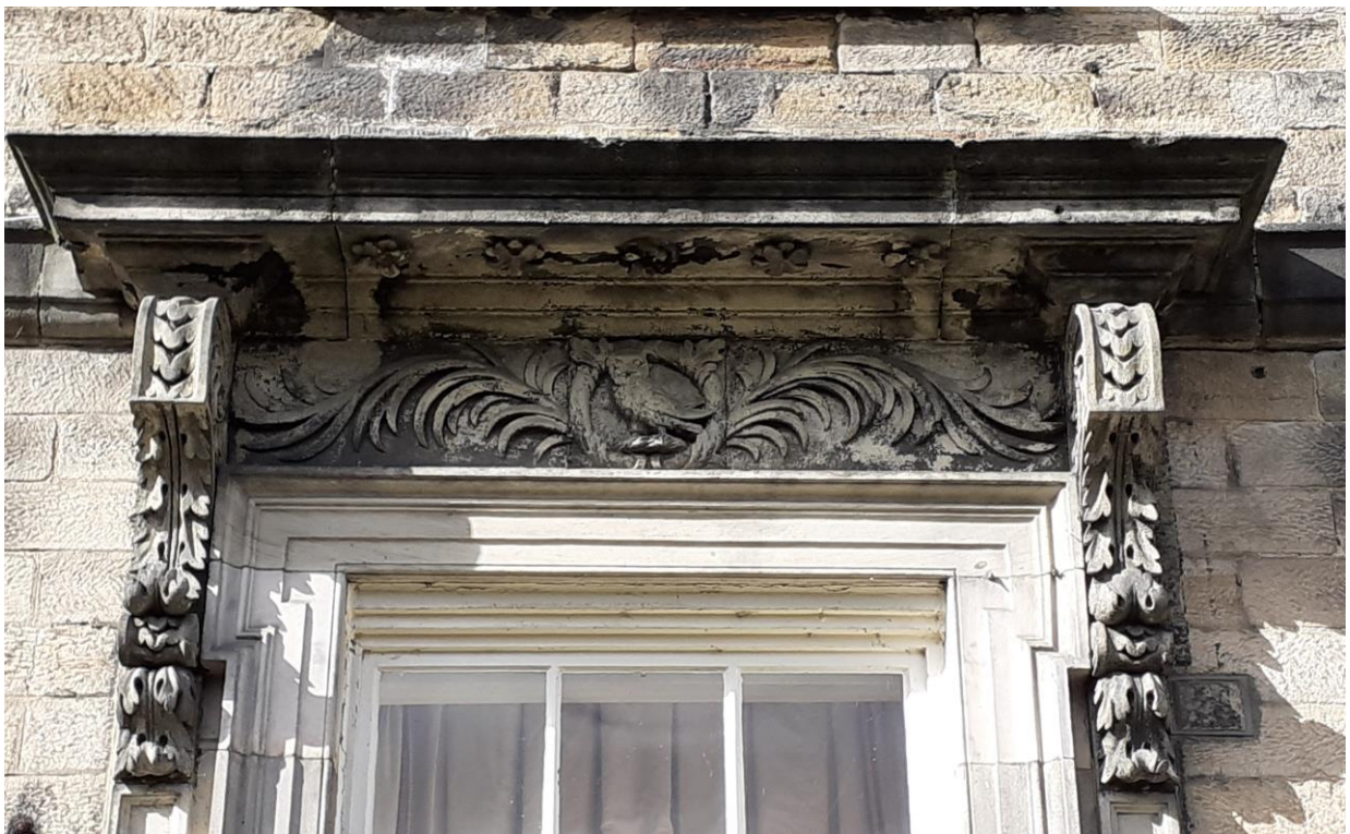
The Calverley horned owl still featured at Esholt hall, here on a lead downpipe and in a door hood.
