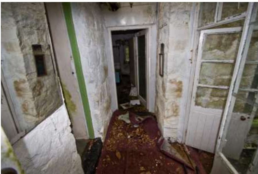
Signs of accelerating decay: the cottage before the main works began.
