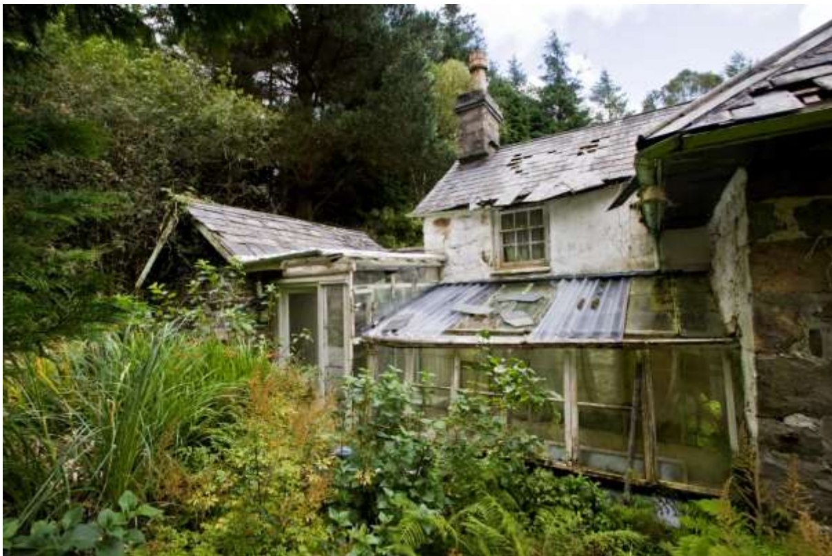
A ramshackle conservatory linked the rear extension to the main rooms. Vestiges of the Johnsons' planting scheme were still apparent.
