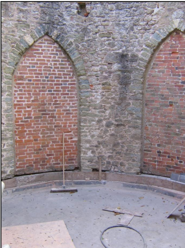
The concrete ringbeam above the kitchen, introduced to prevent this tower spreading.
