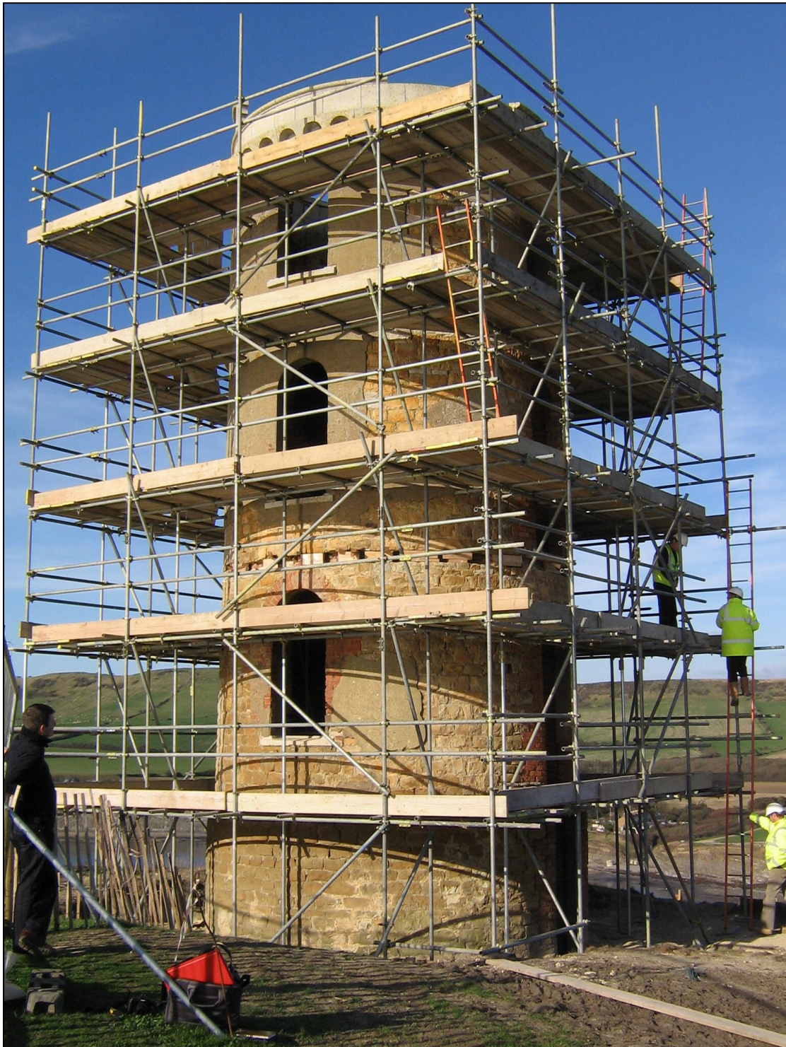
The old tower fully scaffolded, the outer drum by now taken down (summer 2006).
