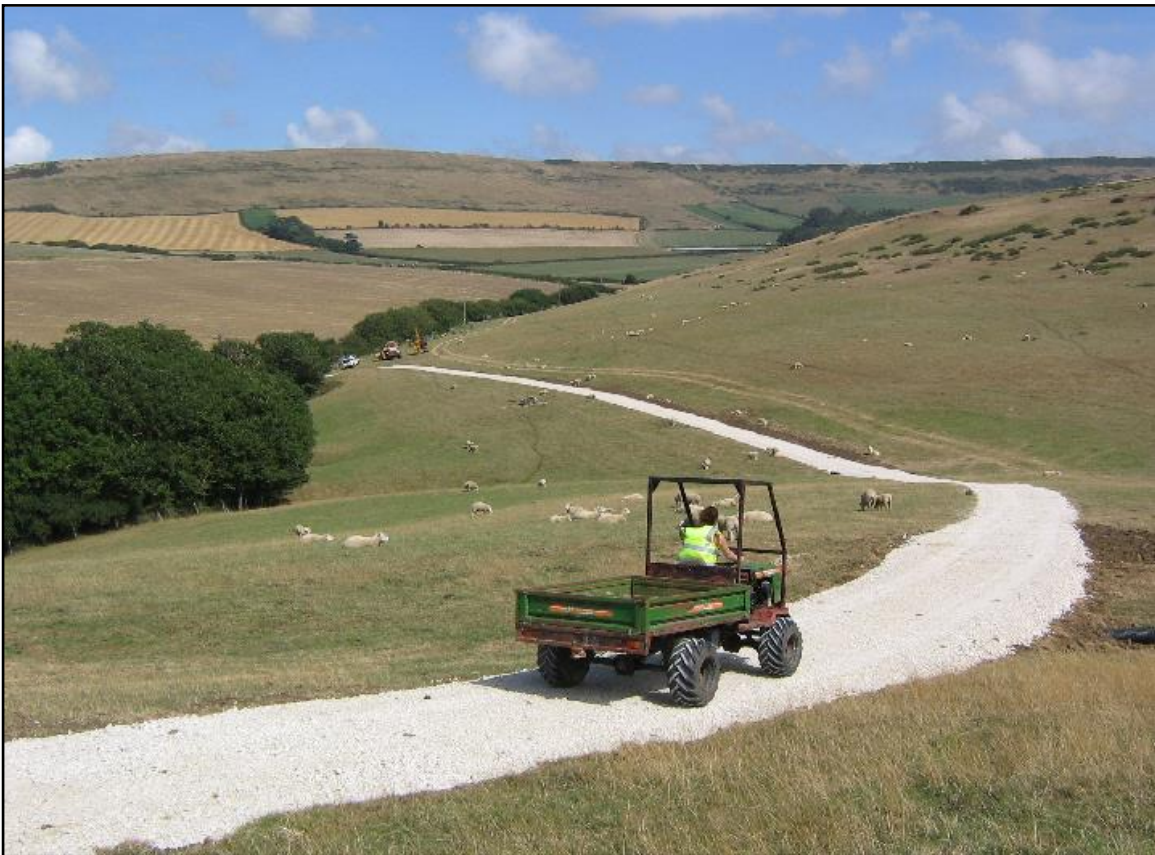
August 2006: the new site access track, leading down to the site office. It would become much muddier before the job was done.
