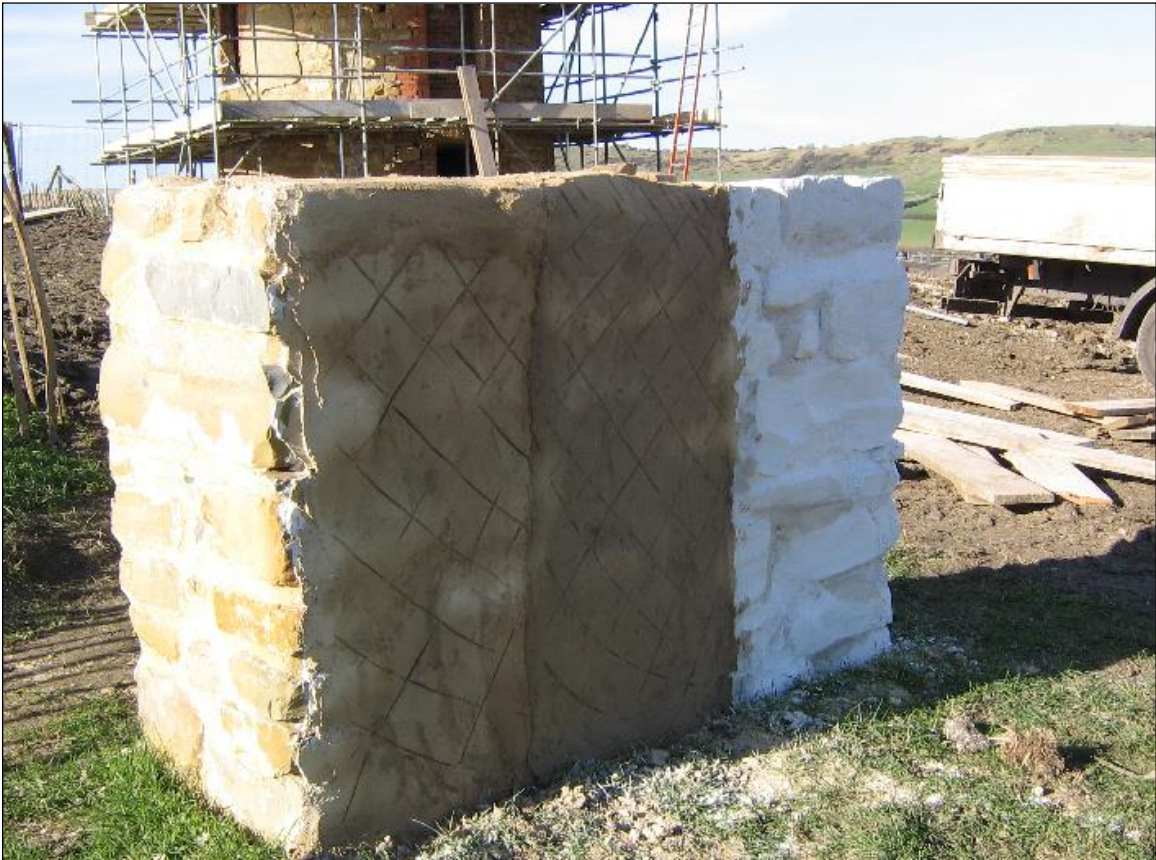
Lime render trials using different aggregates were prepared in August 2006, to allow them to weather through the winter before a decision was made.
