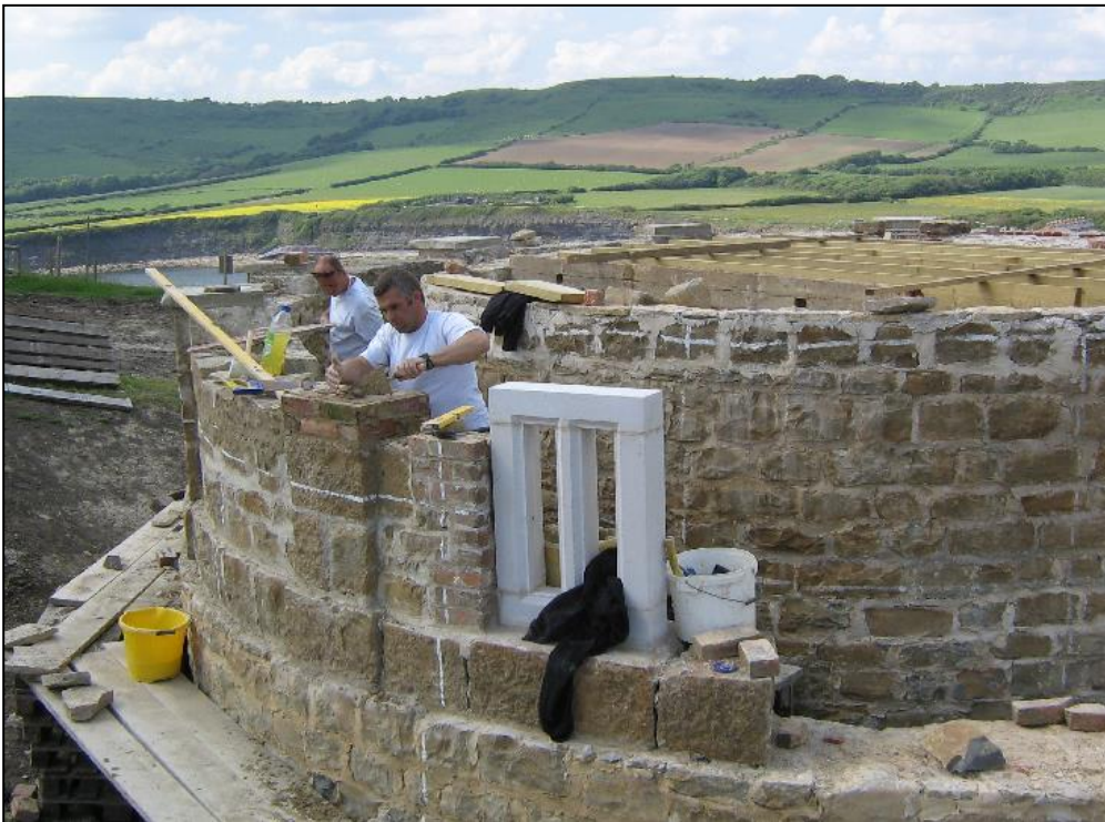
As the new tower went up, the white lines were used to align each quadrant
