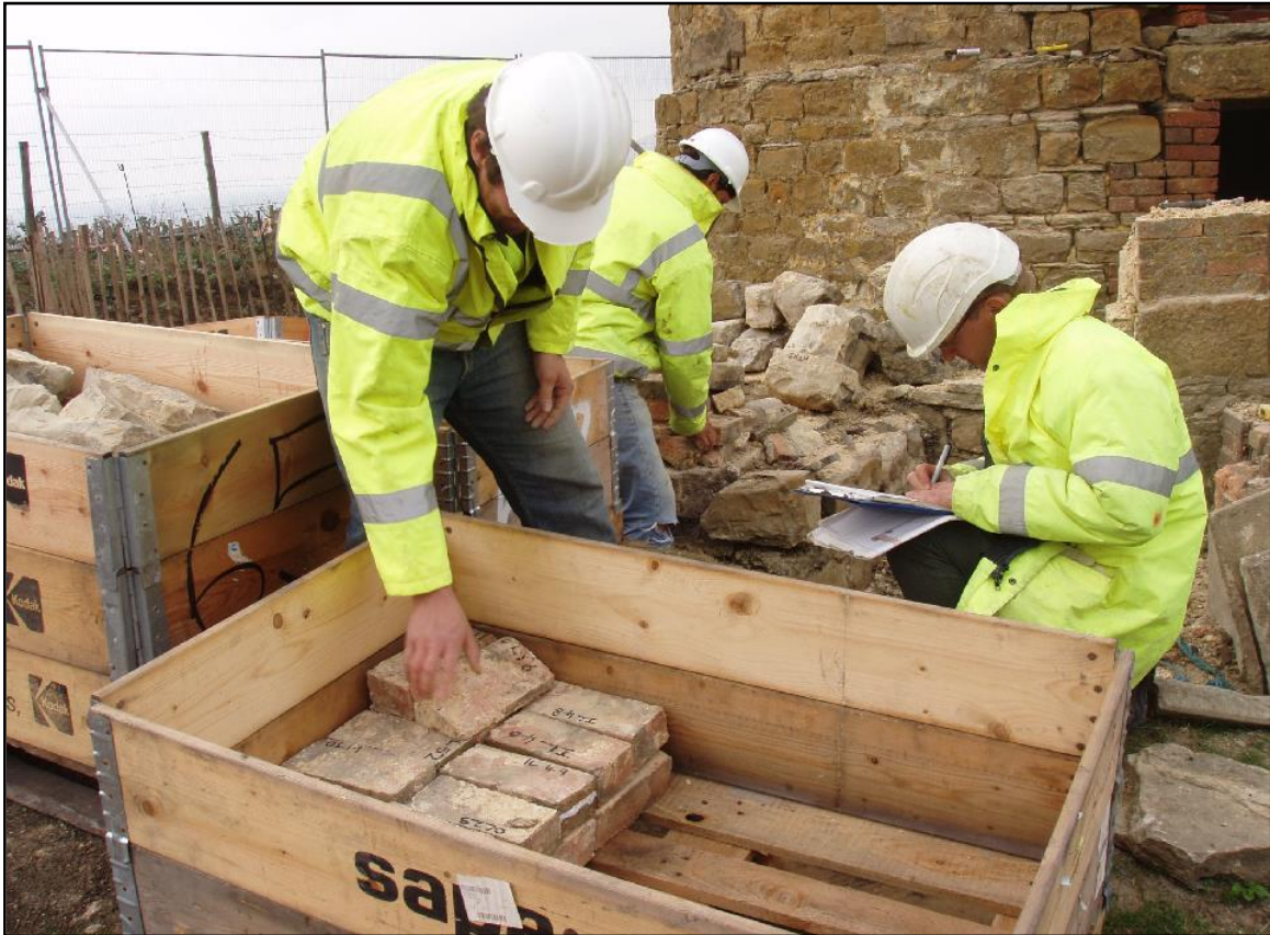
Numbering and recording individual bricks during dismantlement, before storing them in wooden crates (October 2006).
