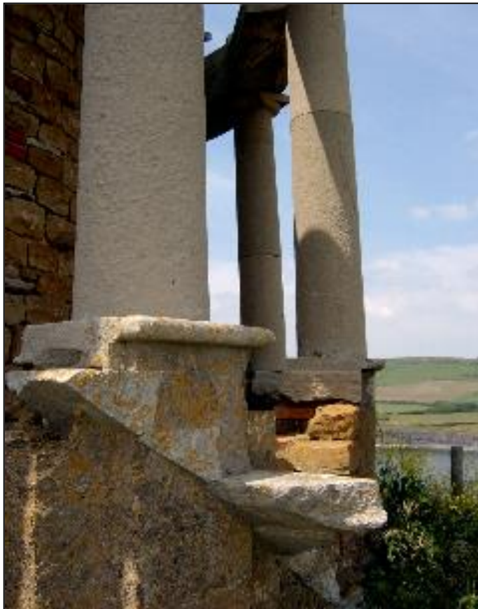
All that remained of the steps.
