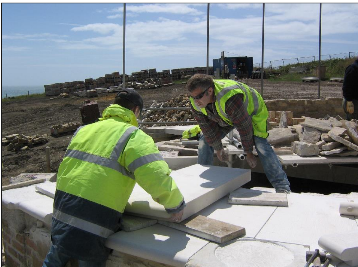
Fitting a new slab. In the background are some of the many crates used to store the numerous pieces of the tower's fabric.
