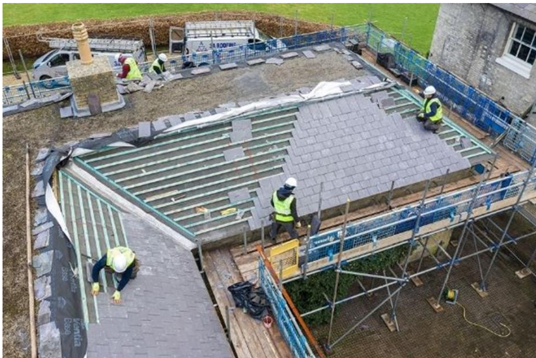
Second phase of re-roofing works underway in 2020-21. Outdoor work ensured that social distancing could be strictly observed.
