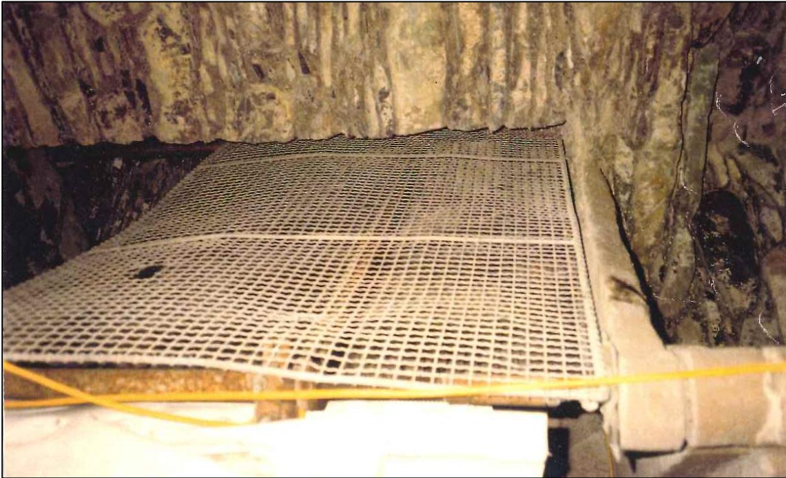
The top steps of the cap house stair were damaged by lightening in 1969 and replaced by Historic Scotland.
