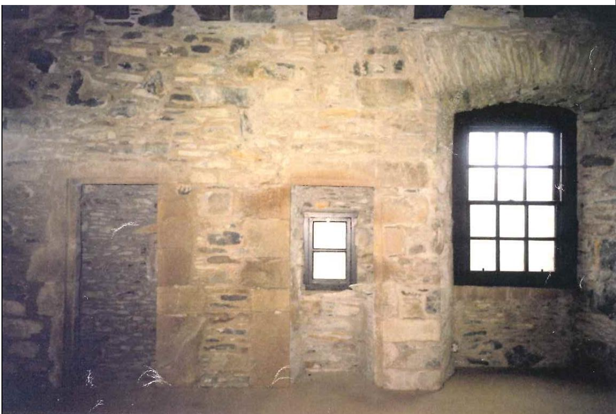
The second floor in 1989. The bathroom wall was inserted between these two garderobes, where it had been originally.
