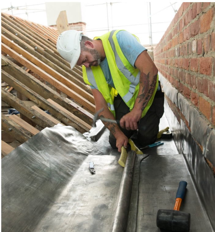
Removal of the roof tiles underway beneath the shelter roof. Note the ill-advised use of polystyrene foam, 'gluing' the tiles down and preventing air circulation, and also the precarious state of the chimney stack.
