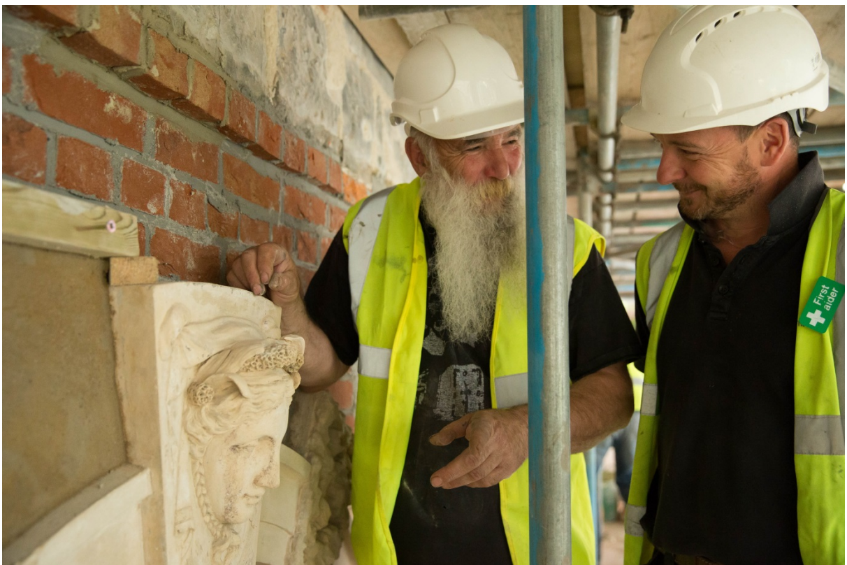
Coade stone craftsman Philip Thomason and Site Manager Stuart Leavy share a joke as they reposition Amphitrite after the repair of the northeast corner.
