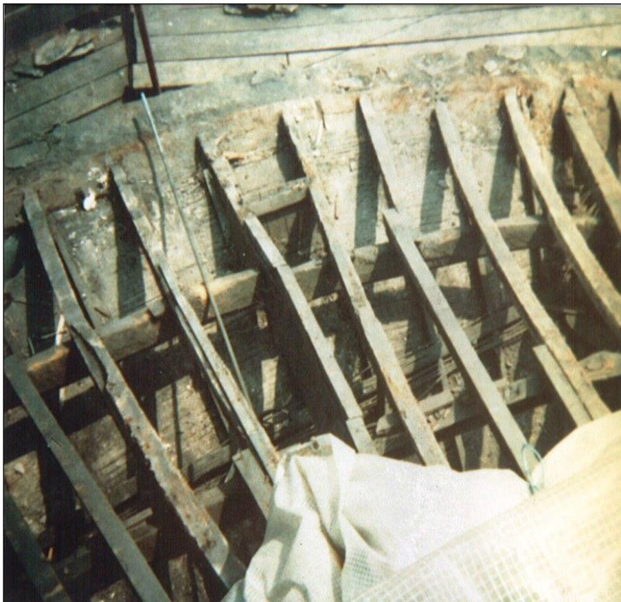
Looking down on the main, lower, roof. Its construction consists of principal rafters running from an outer wallplate to the upper section of the inner drum; trussed purlins curved to follow the line of the walls; and common rafters.
