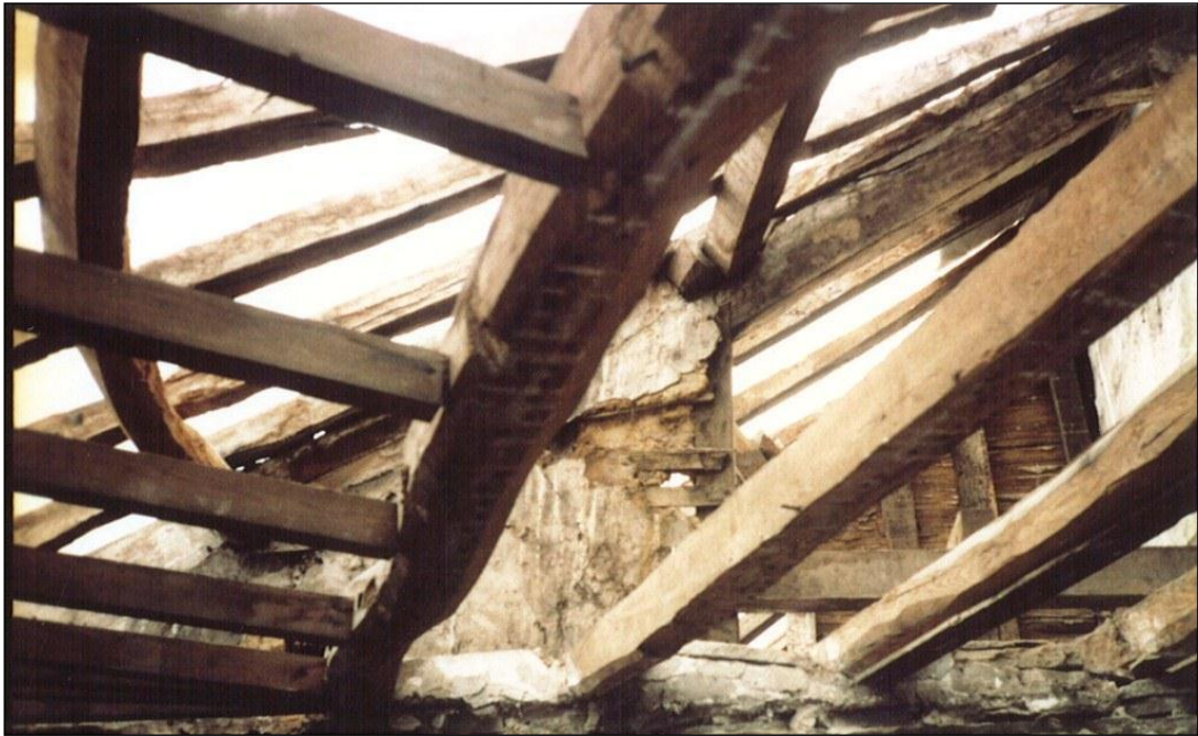
Looking at the roof from inside the almshouses with the ceiling taken down. Posts to support the principal rafters can be seen resting on the radial partition walls.
