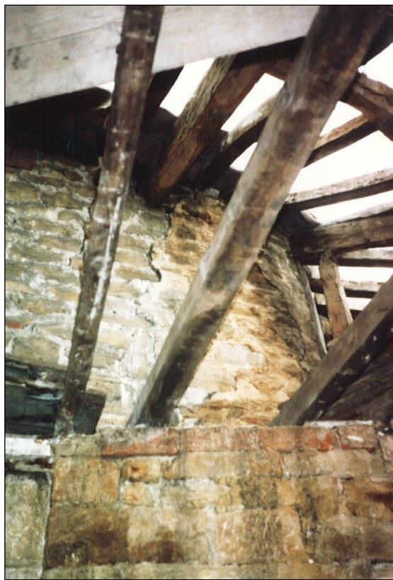
From the mother's room; showing how the ends of the principal rafters are built into the upper section of the inner drum.
