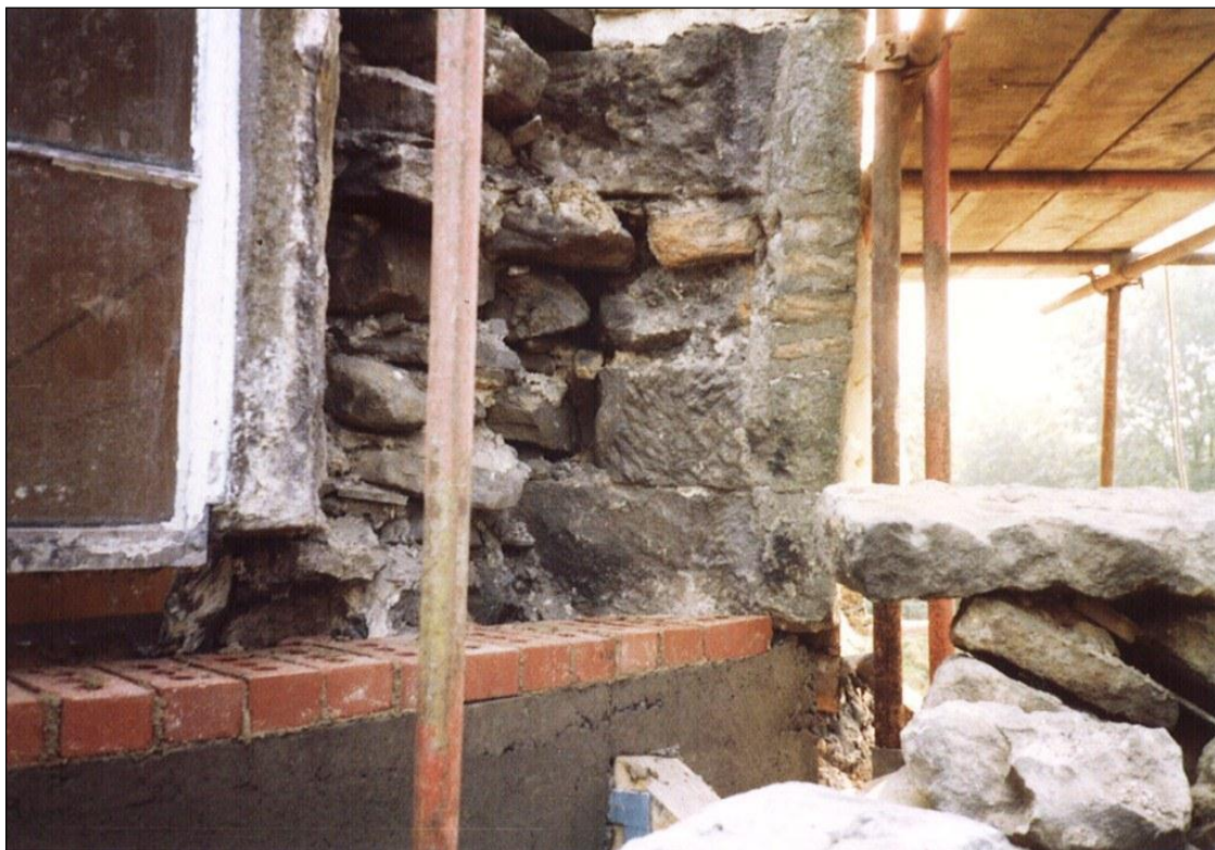
A ring beam was formed round the inner drum to hold the rafters of the main roof. The end of one can just be seen built into the new work.
