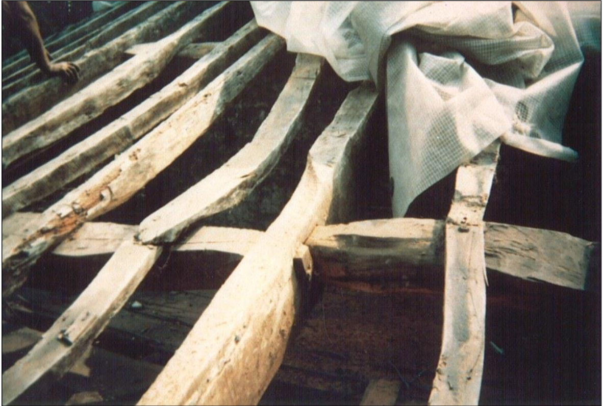
Main roof: principal rafter, purlins and common rafters before repair.
