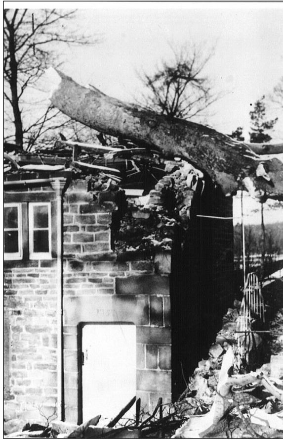
The laundry after a tree had fallen on it in 1969. It was afterwards demolished.
