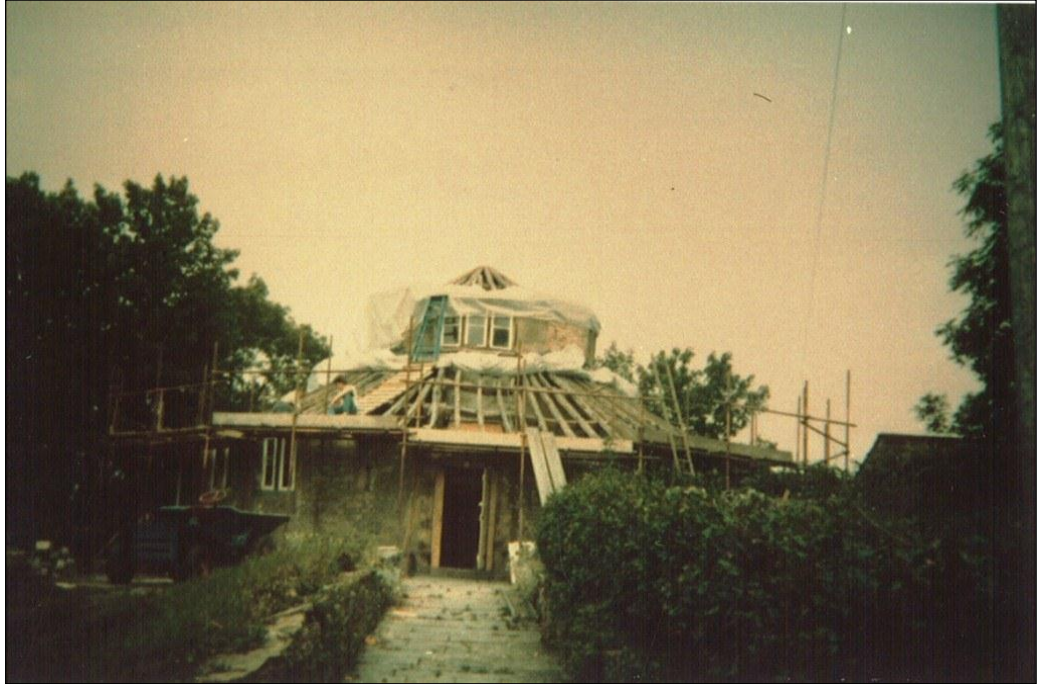
The roof stripped of its slates and with the chimney stacks taken down.
