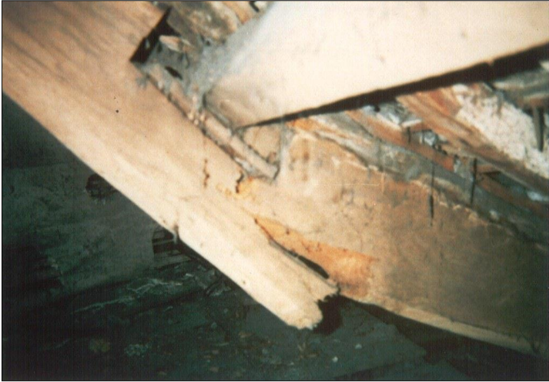
A broken principal rafter. Only one principal rafter had to be replaced, above the dining room. The others could either be repaired, or were sound.
