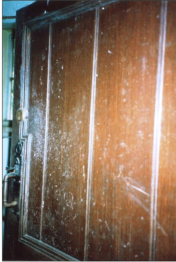
The doors were painted in 'grained oak colour' in 1810 and probably before.
