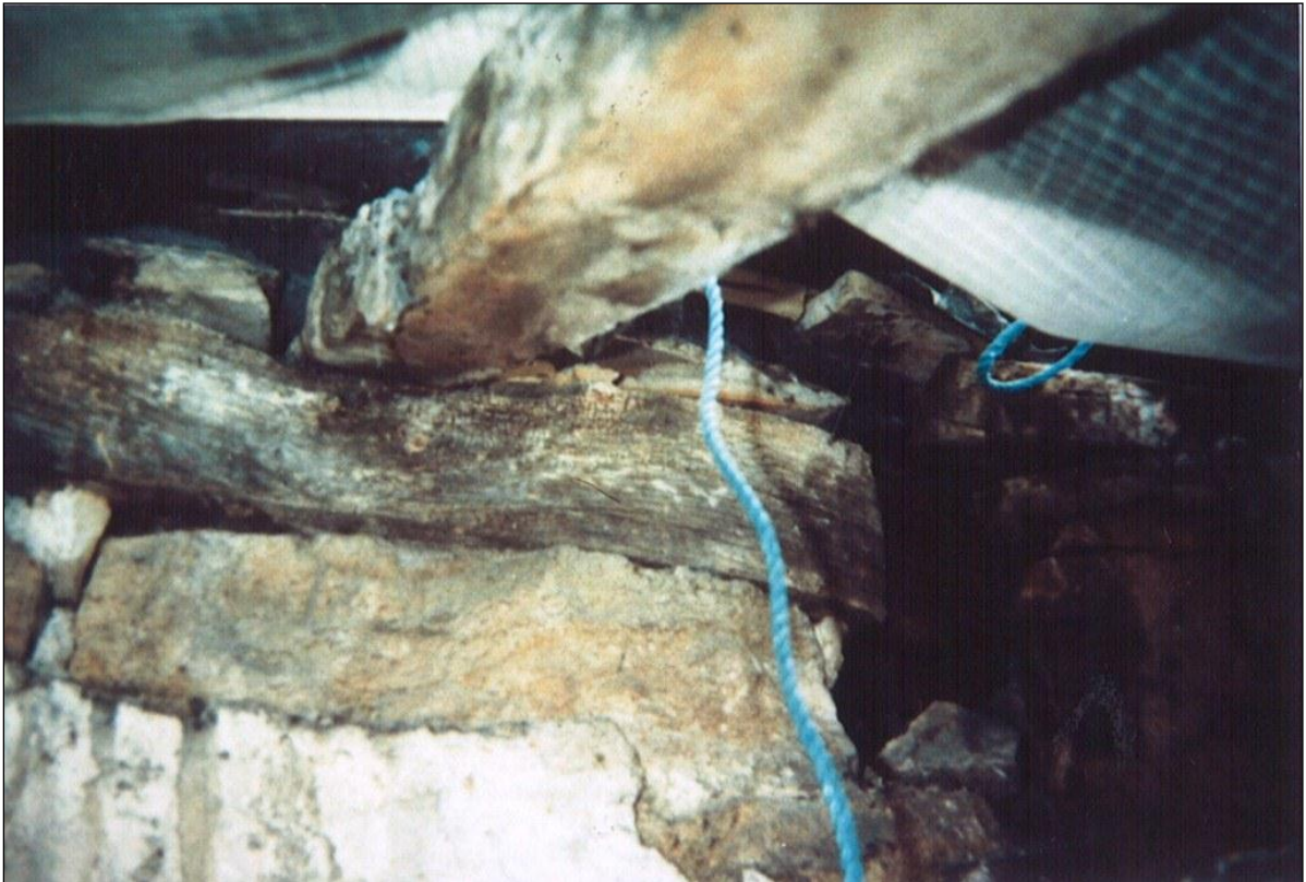
Bearing of rafters of lower roof against masonry inner drum, before repair.
