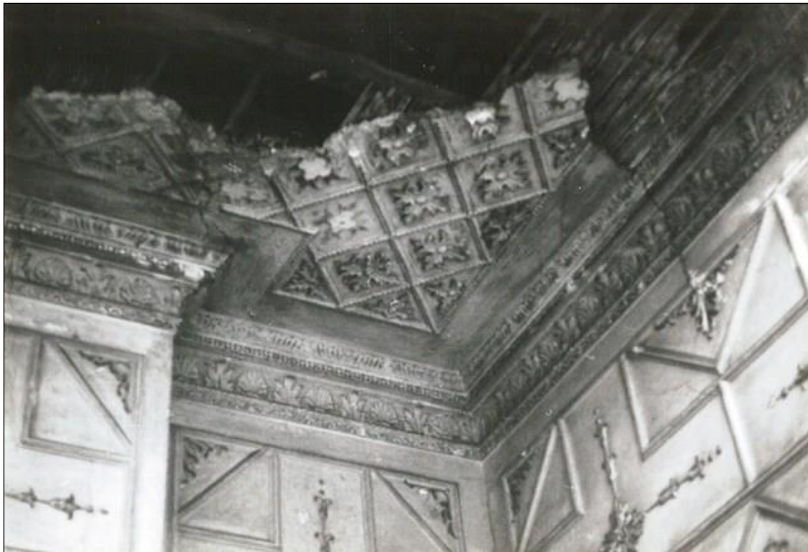
The decorative plaster ceiling in the bedroom which collapsed and was not replaced.
