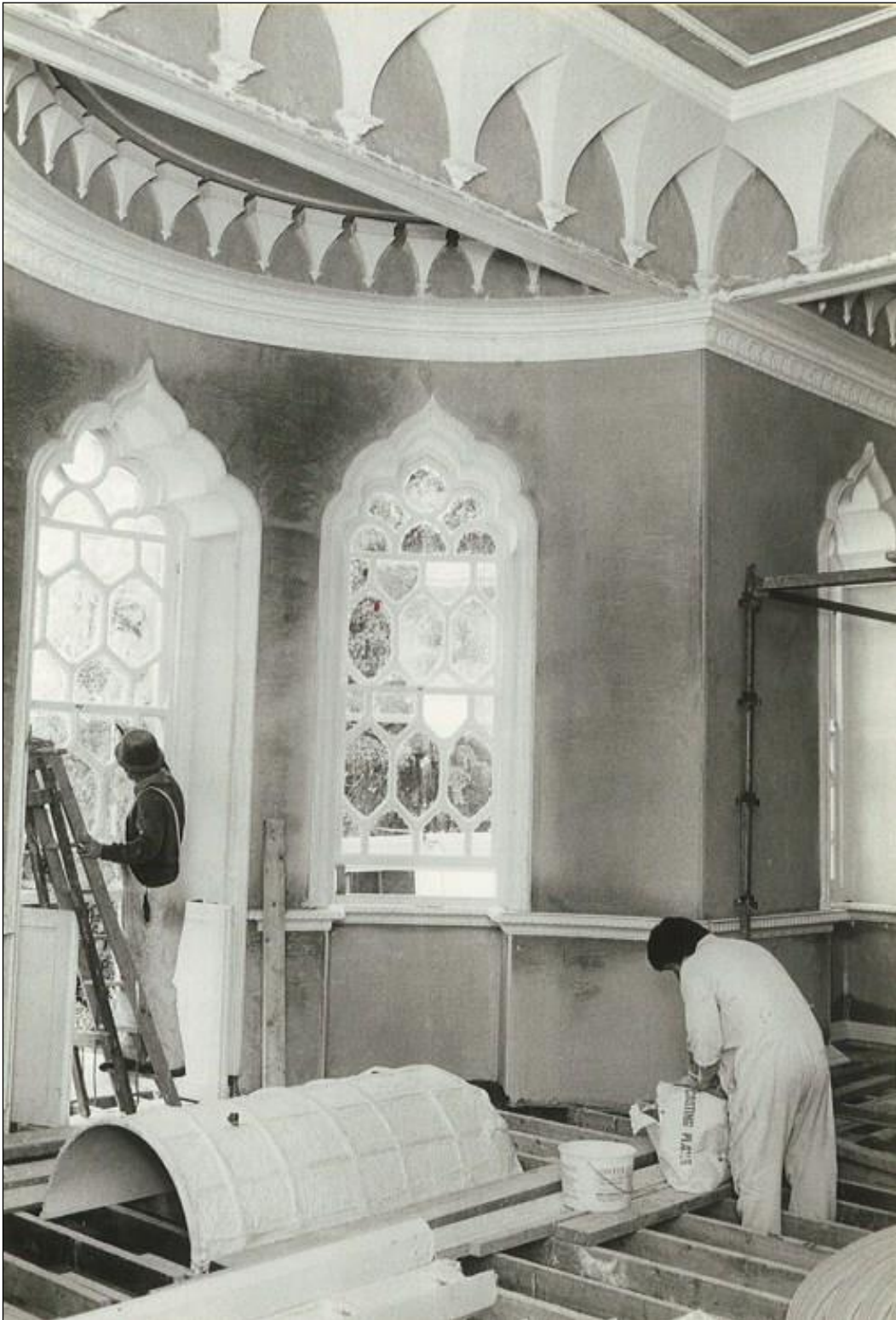
The Banqueting House nearing completion. The floor was put in last. It is pine like the original and the boards are 7½" wide. The chimney piece was discovered buried outside the building. Part of it was missing and Mr Stoker carved the head on the right hand side roughly to match the existing one. Mr Greenhill, the painter, is on the left. (Gateshead Post)
