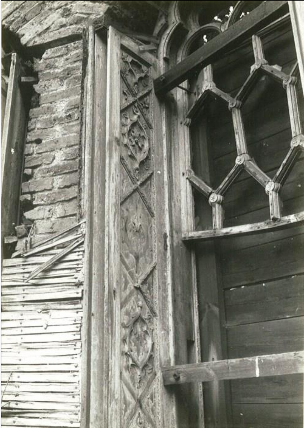
One of the shutters in the Banqueting Room. The carving from the six remaining broken shutters was removed and then pieced together to make a single complete pair, now in the bedroom.
