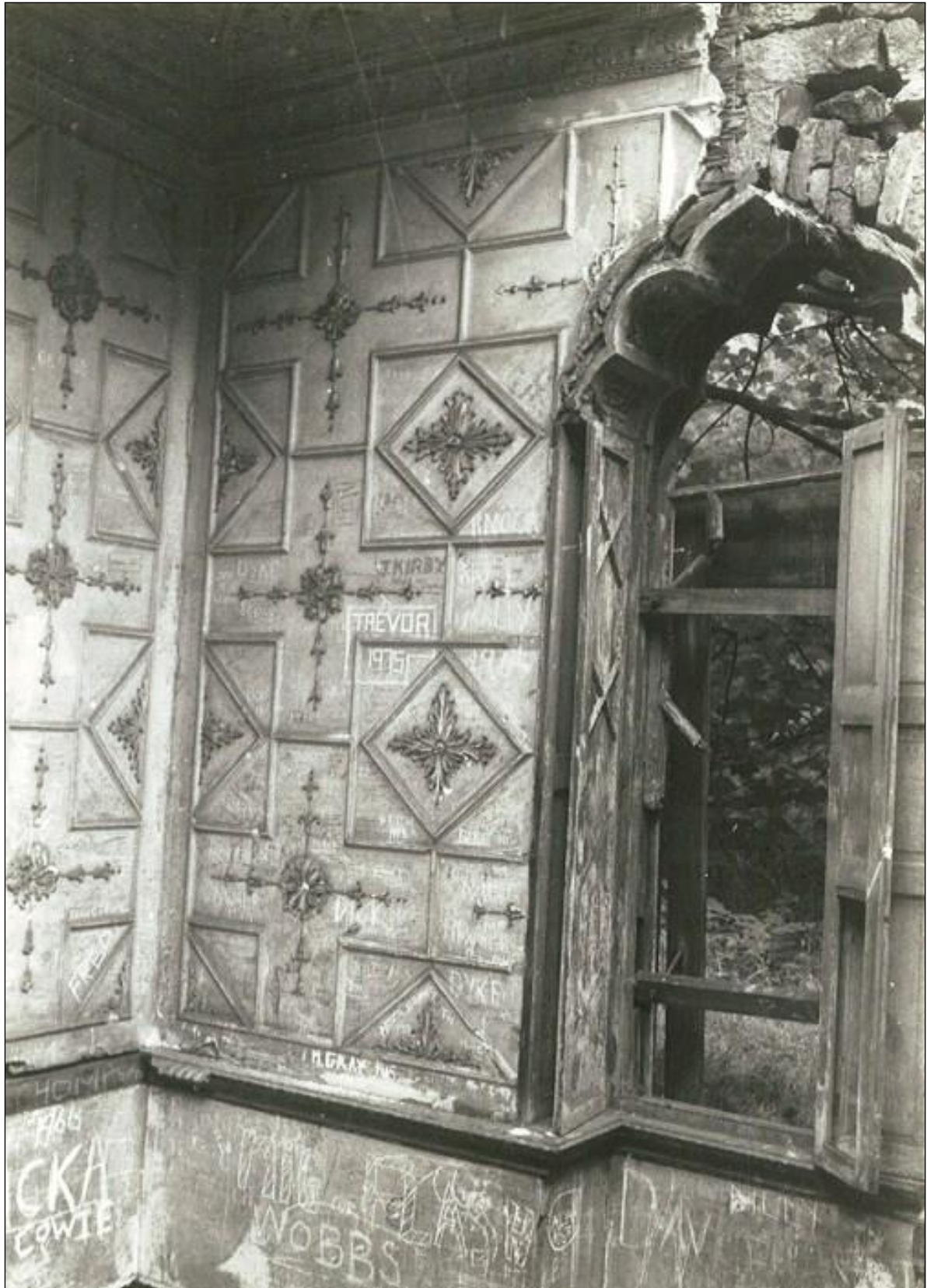
Most of the plasterwork on the bedroom wall with the window in it, is original.
