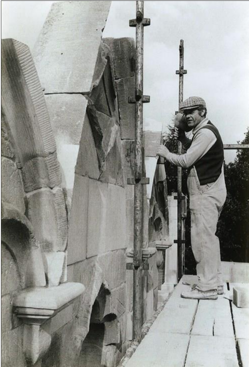
1980 Work in progress. Mr Stoker, the mason on the roof (Gateshead Post)
