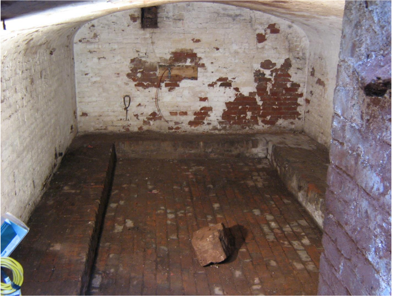
The Victorian cellar underneath the hall. The shelf is for barrels of beer
