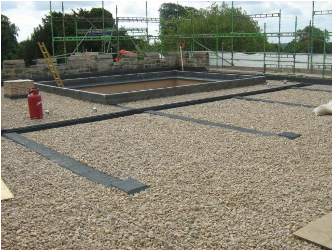
Gravel ballast to the upper roof laid over an insulated membrane system
