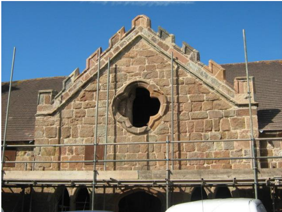
Len Hardy's rebuilding of the front of the Coach House nearing completion
