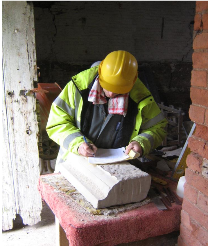
John Brown carving a replacement drip mould stone for the front elevation
