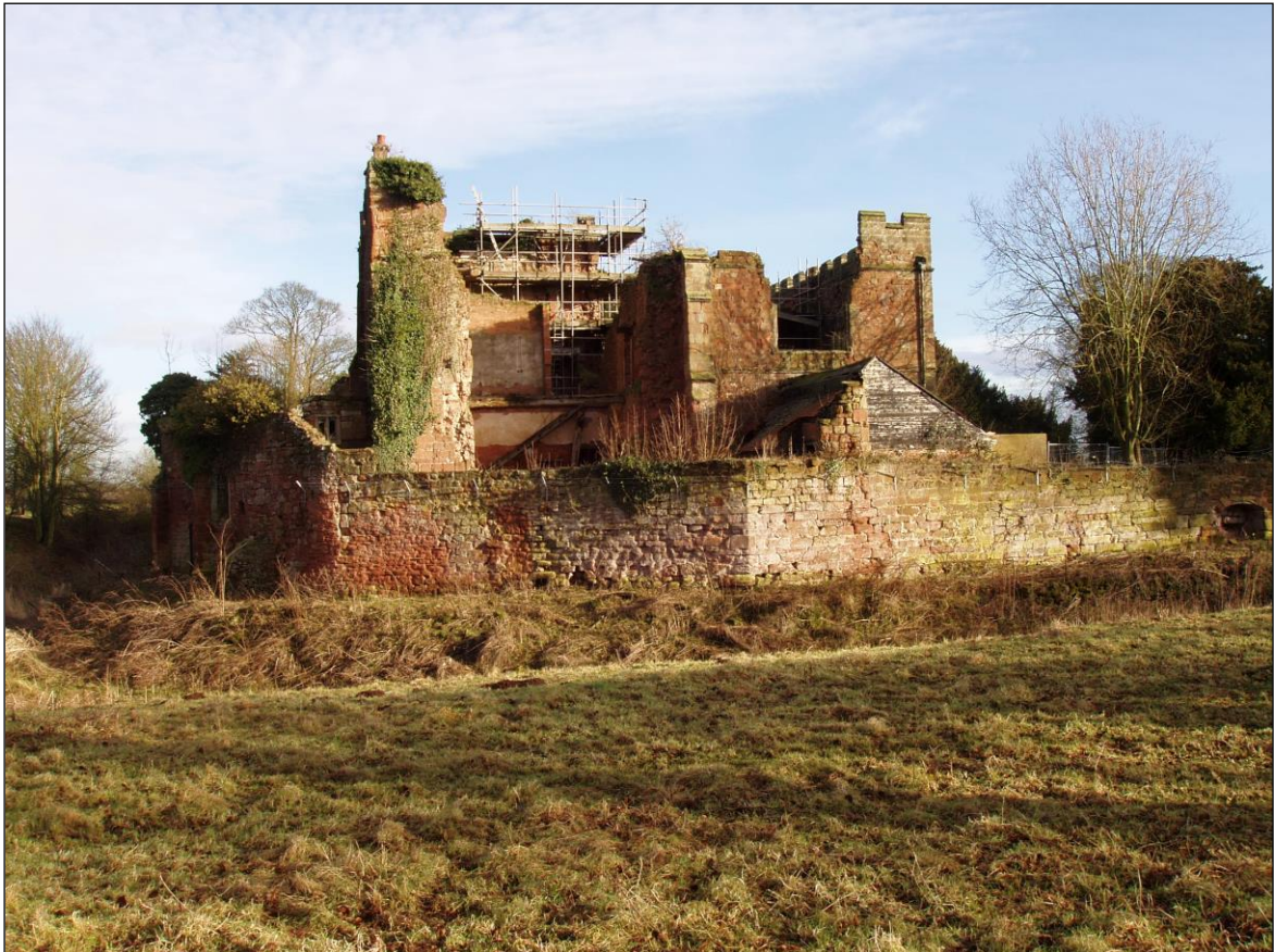
The same view in 2005 with much of the south elevation now collapsed
