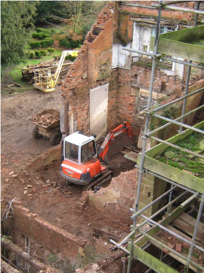
Top: Clearing out the N end with a small digger and dumper truck after the taking down of the N gable.
