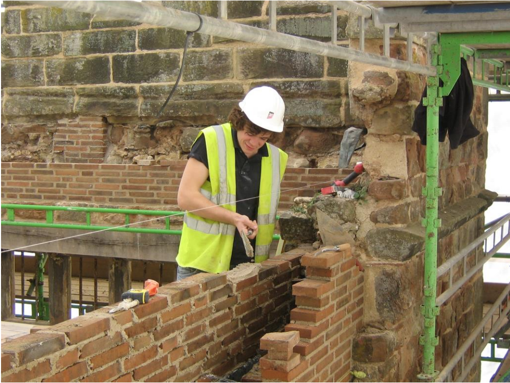
Nathan Grassby lays new brickwork at the south end of the garden court
