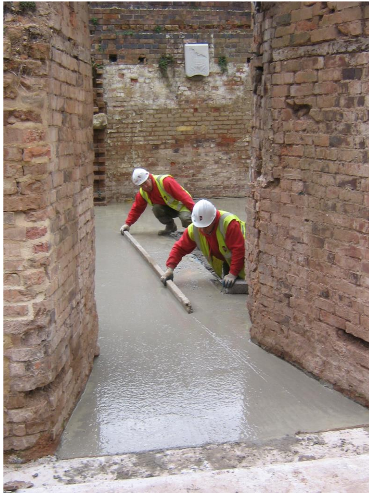
A new floor slab being laid. A 'bat box' is on the rear wall
