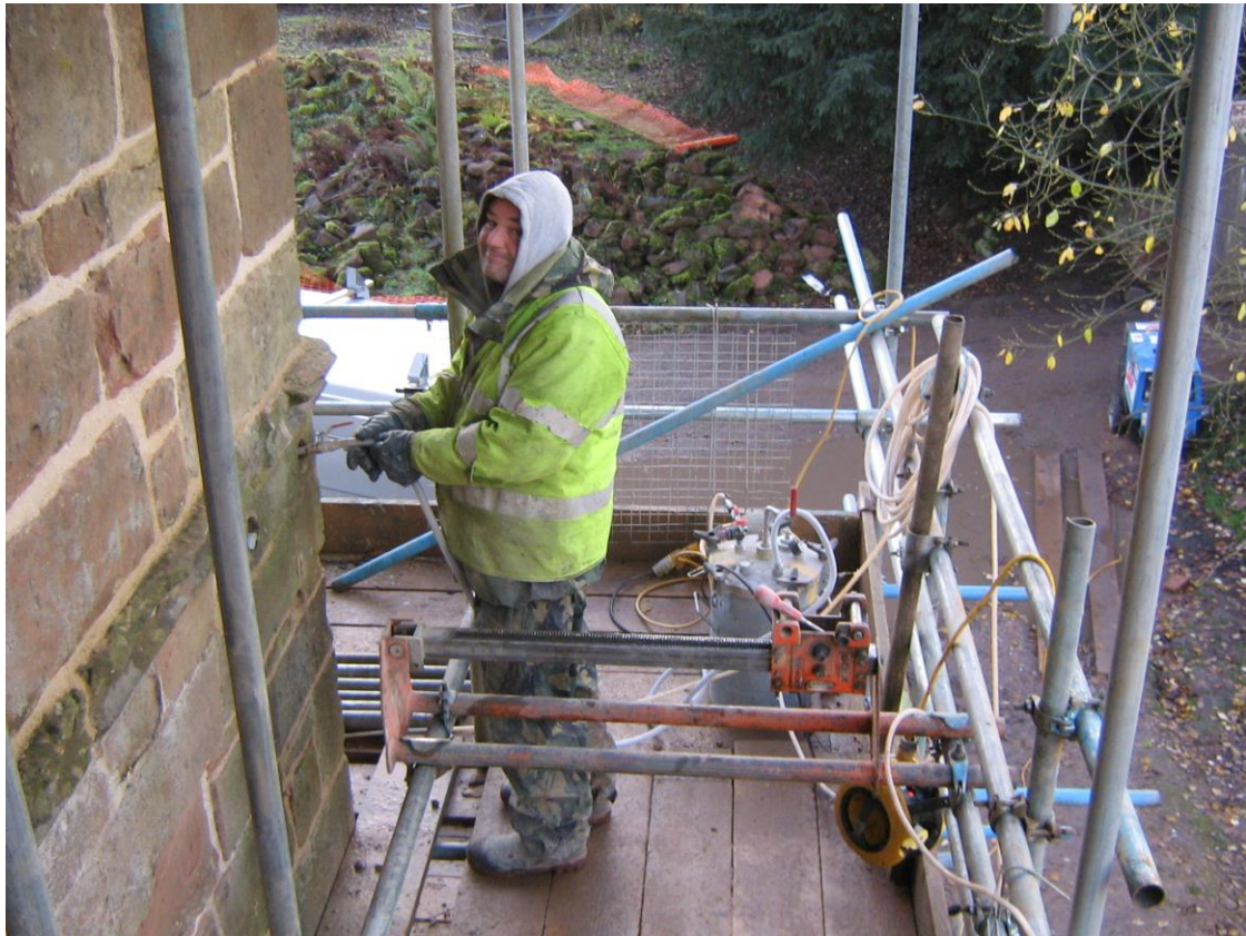
Pumping grout into the two 11m long anchors inserted into the SE corner
