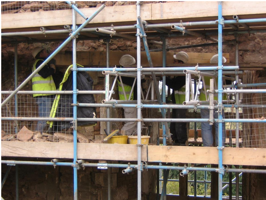
Manhandling one of the new oak lintels into position on the west wall
