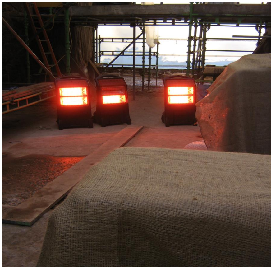
Heaters were needed to keep frosts at bay and thaw out pallets of bricks
