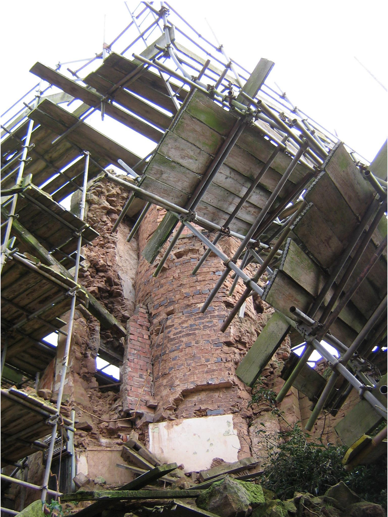
Most of the vice had collapsed by 2007 leaving only a thin brick inner lining. Its remnants now hold the lift.
