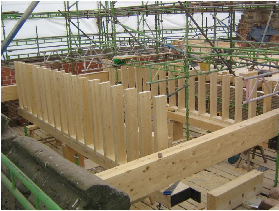
The principal glulam beams and joists to the courts start to take shape
