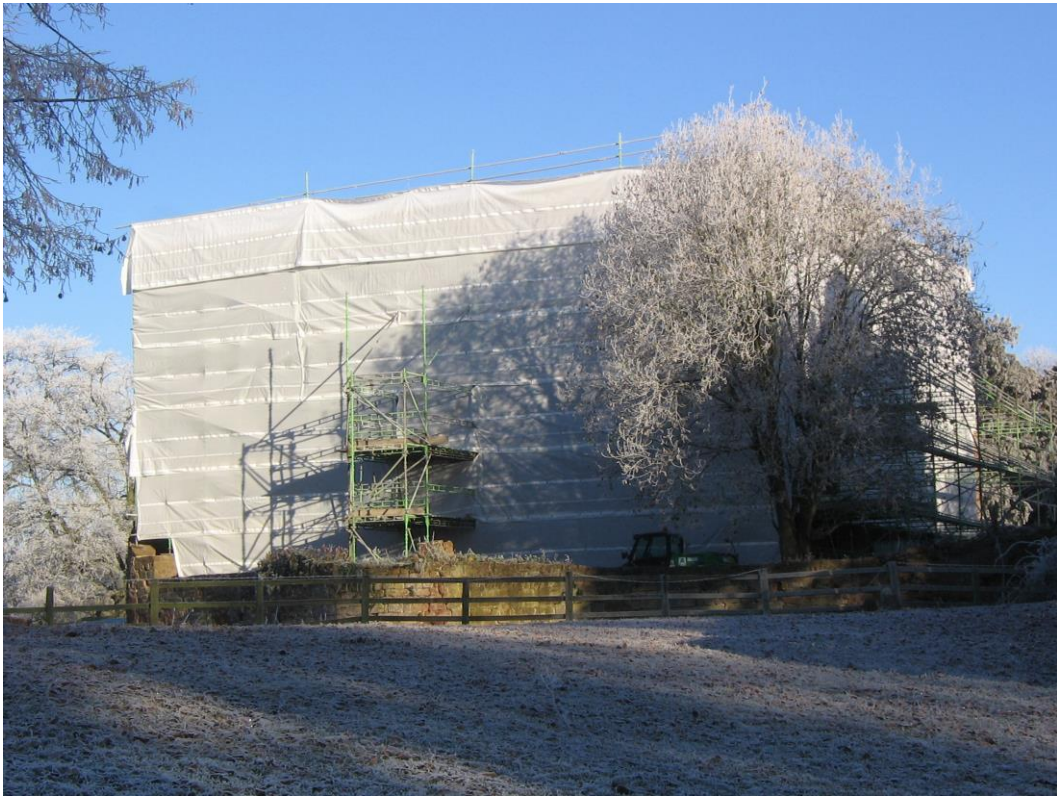
Fully scaffolded with a loading bay, Astley endures yet another cold winter
