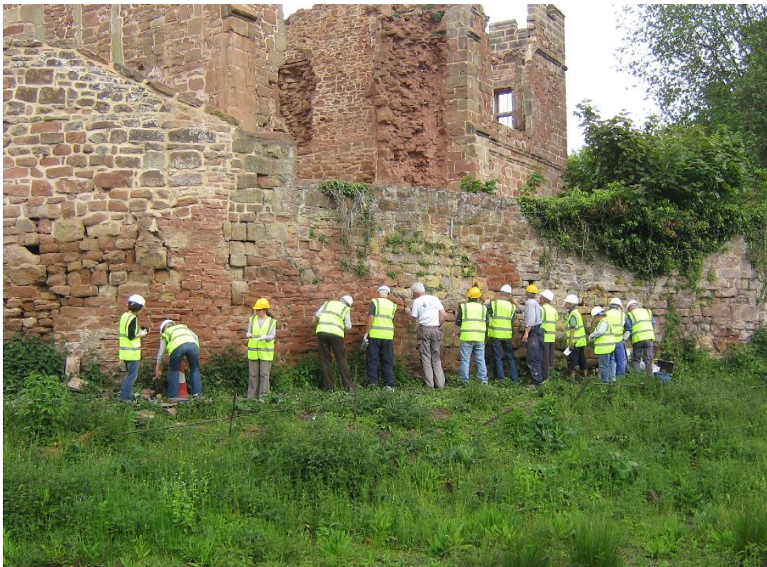
John Brown runs a day on lime repointing for volunteers and Landmark Friends, making a real contribution to the repointing of the curtain wall.
