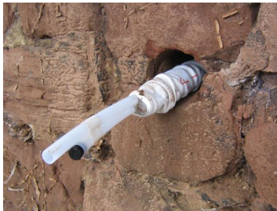
A Cintec anchor in its drilled hole before it has been pumped full of grout
