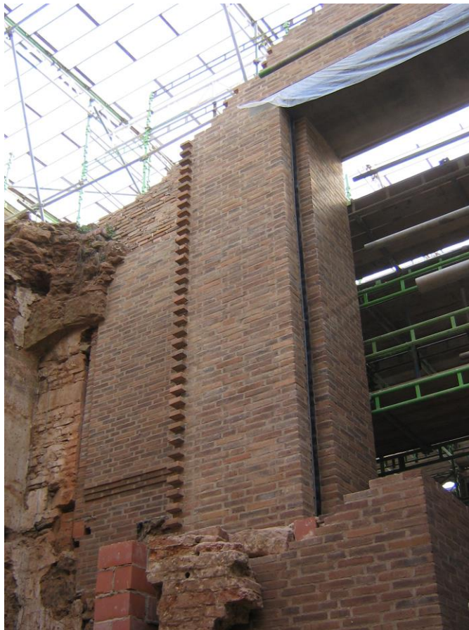
With some scaffolding down, the scale of the new brickwork becomes apparent
