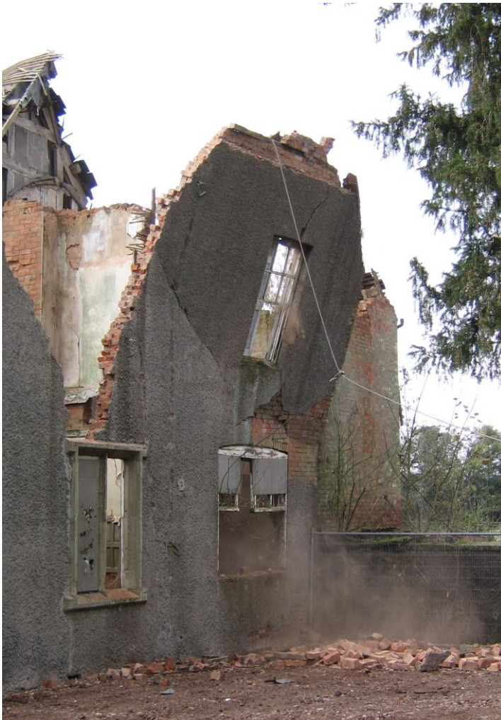
Above: looking down into the south west corner of the castle, site of today's living room, from a cherry picker before work began.
