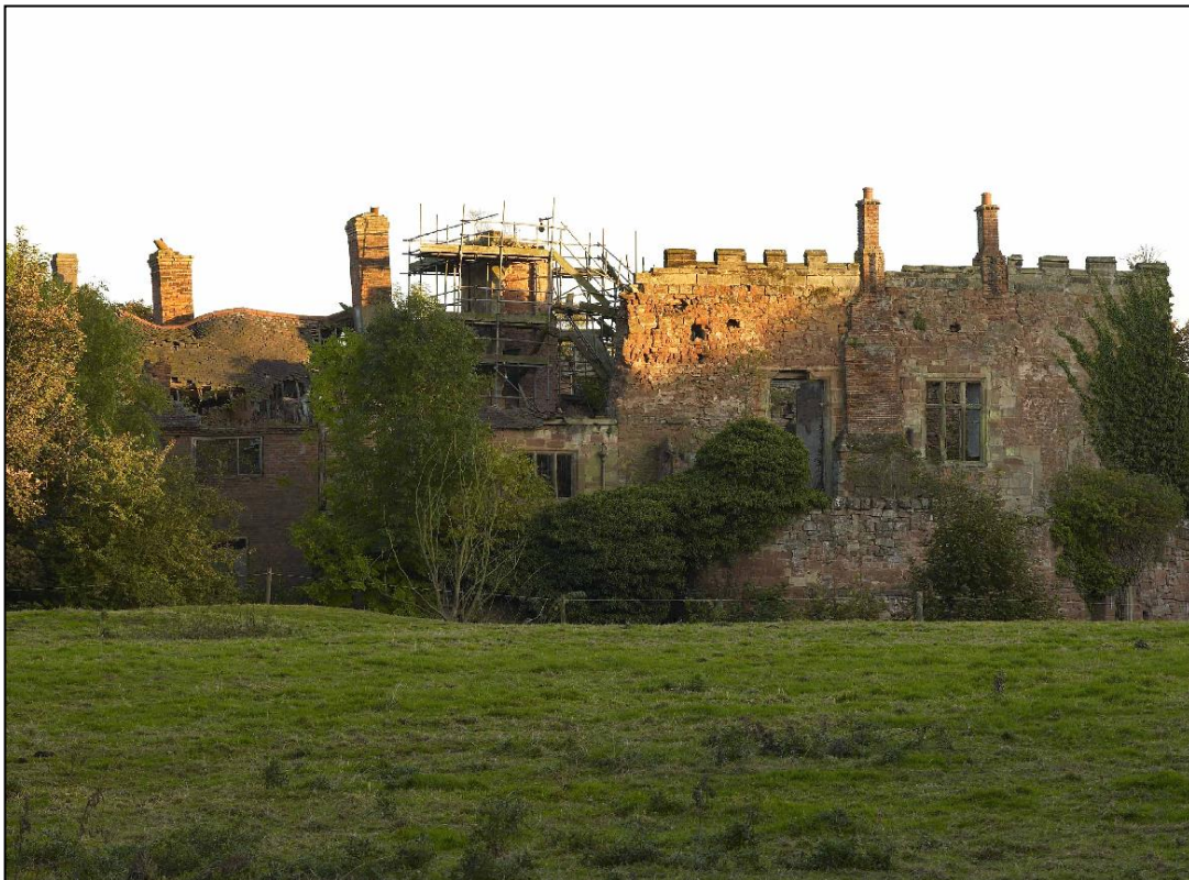
East (top) and west elevations of Astley Castle in September 2007. Note the inner skin of the vice tower still standing in the centre below, and the northern portions of the castle that could not be saved and had to be taken down.
