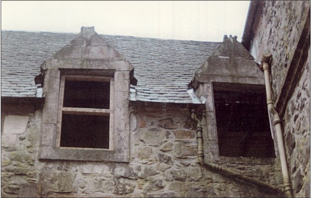
The East dormers and old drainpipes. The date is just inside on the right hand dormer.
