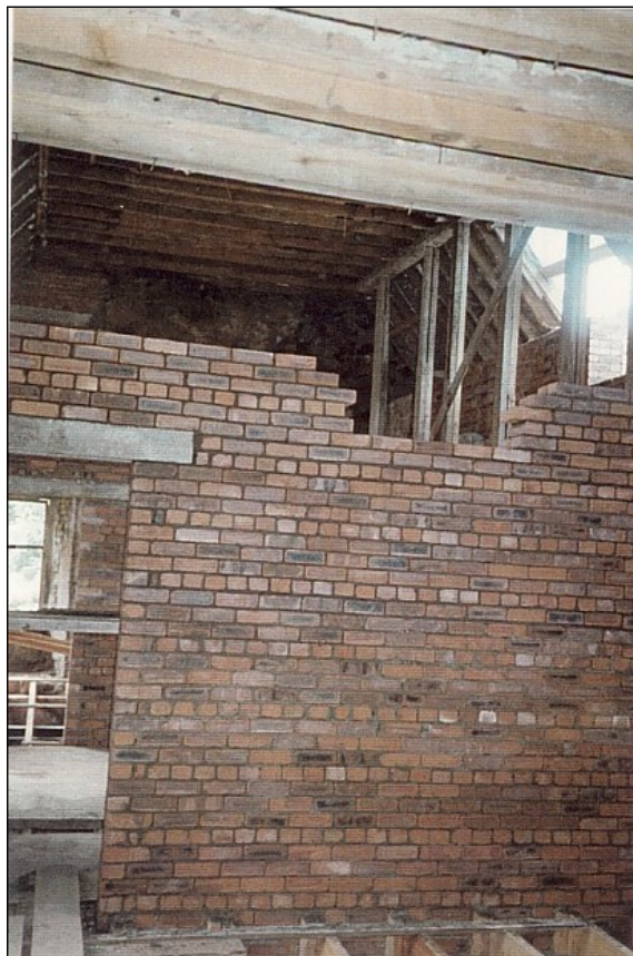
New structural brick walls tying the front and back of the building together.
