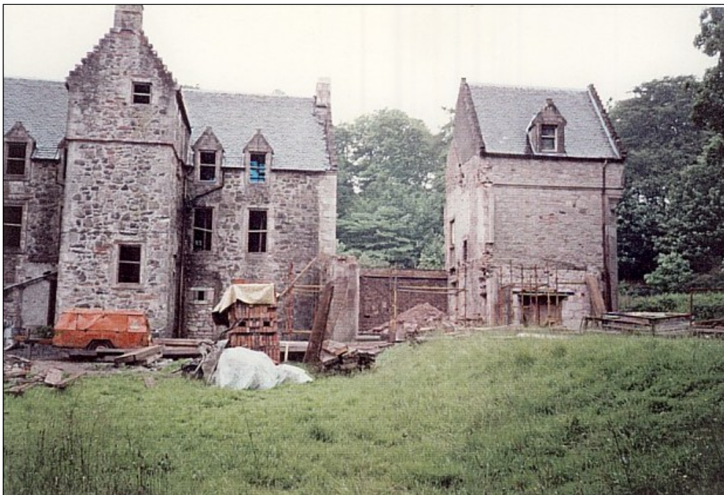
The entrance front after the demolitions. Note the lower ground level in front of the old house.
