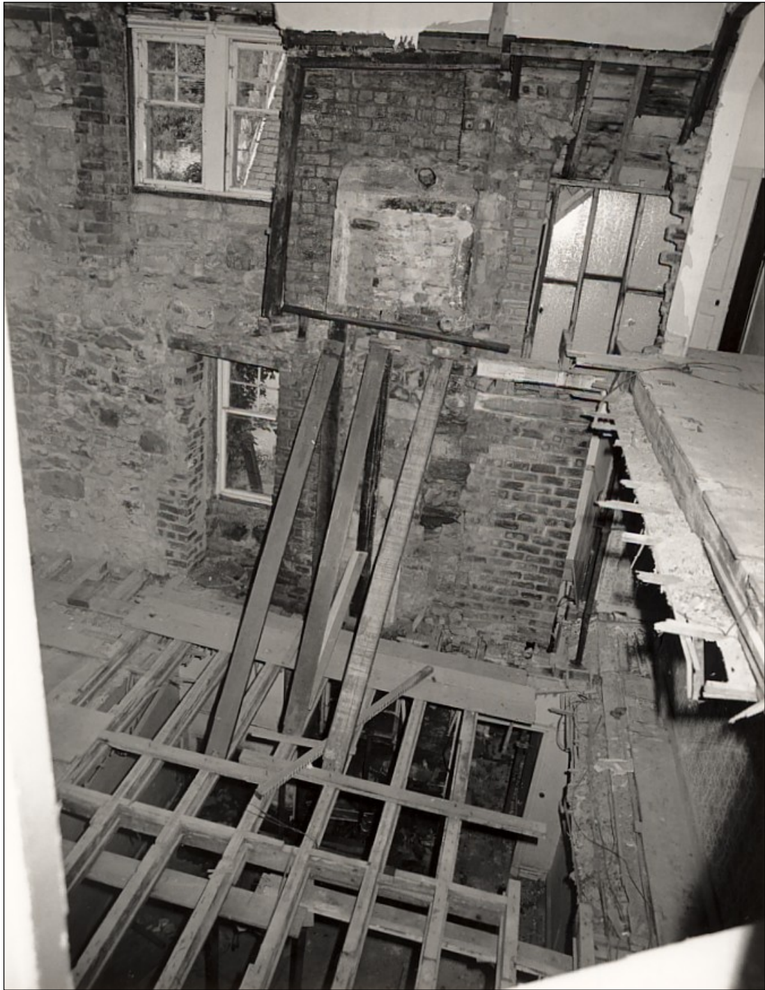
Inside the old house in 1989, looking west. The west wall was shored up inside as well as outside, and the floors had gone.
