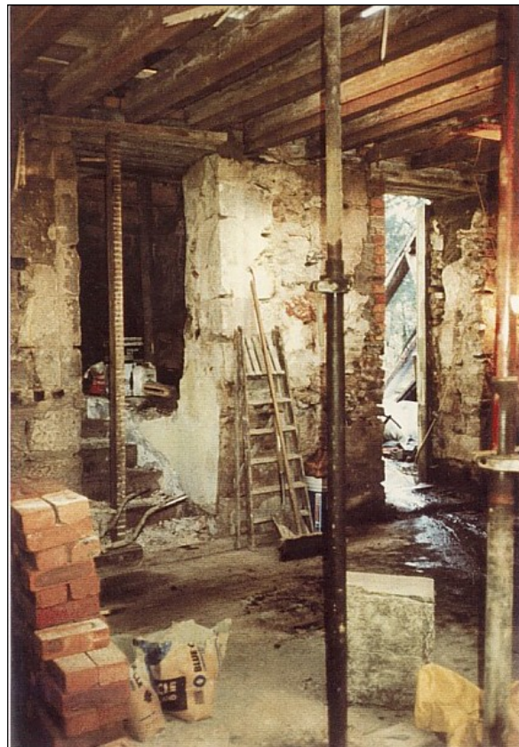
The basement with the 19th century front door on the right. Stairs up to the original (and present) front door on the left. They were full of dry rot.
