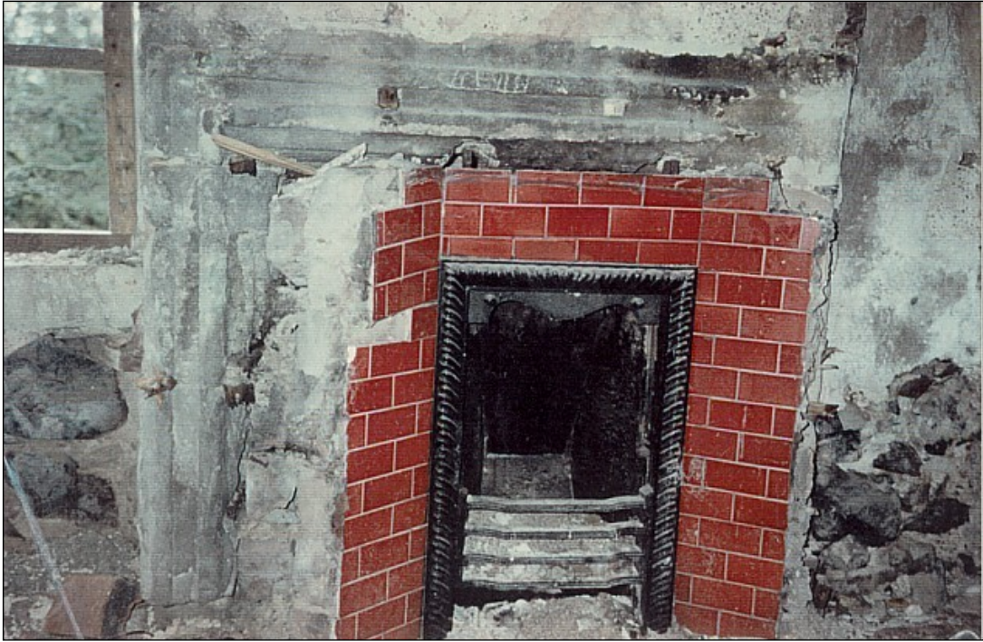
The Victorian fireplace which was in front of the older one in the cap-house, which has now been repaired.
