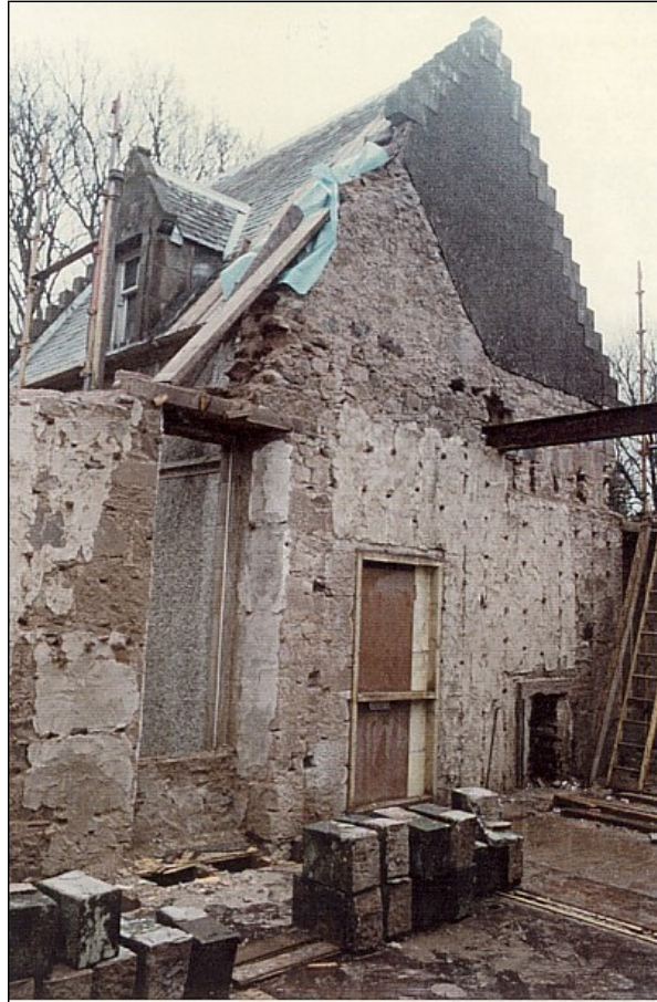
The Victorian stair tower, still attached to the rest of the house.
