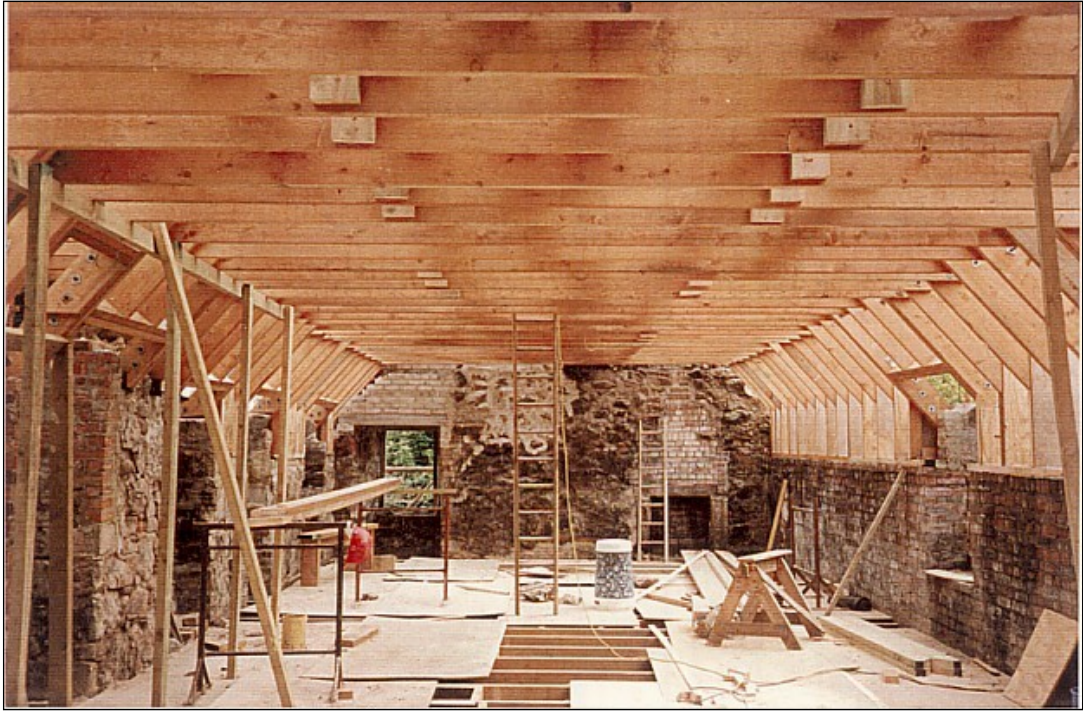
Bedroom floor looking South, showing the new roof structure, copied from the old timbers destroyed in the fire.
