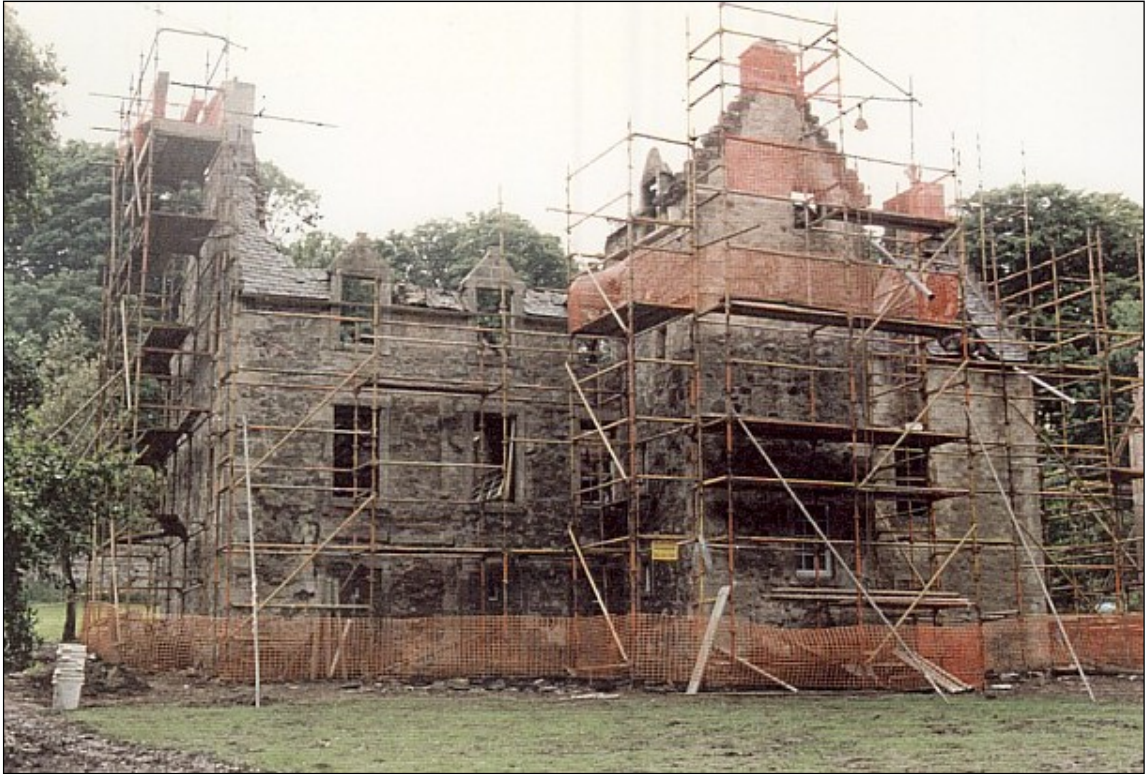
The East front after the fire in June 1991.
