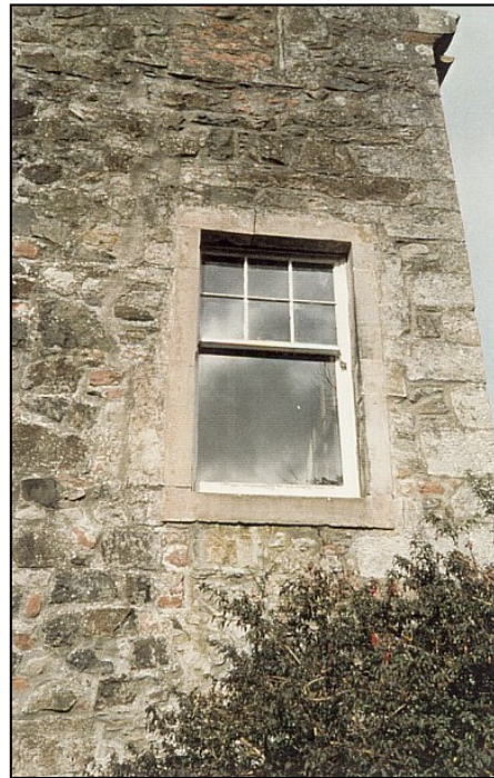
Blocked second floor window on the south end. The cracked lintel of the first floor window was repaired.
