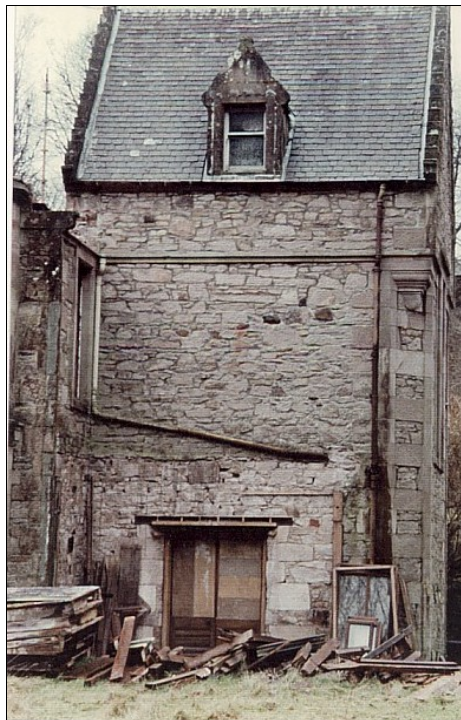
The last of the front doors, leading into the north side of the stair tower.
