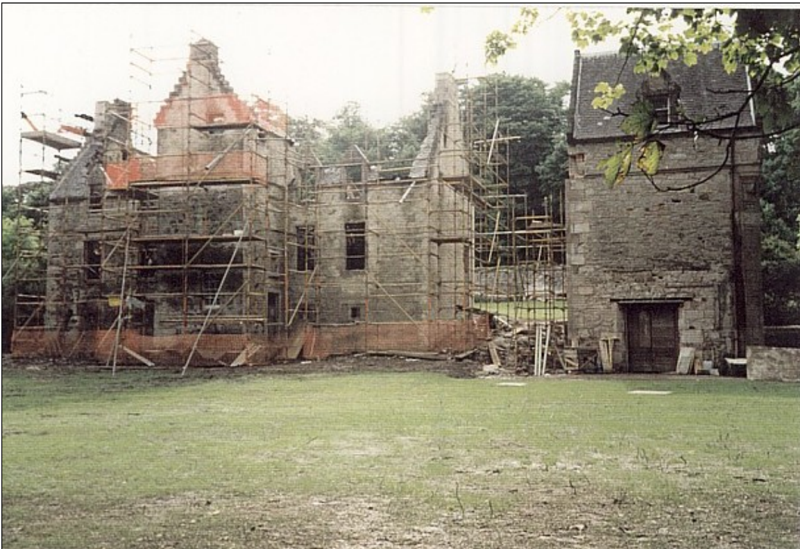
After the fire. The stair tower was untouched.
