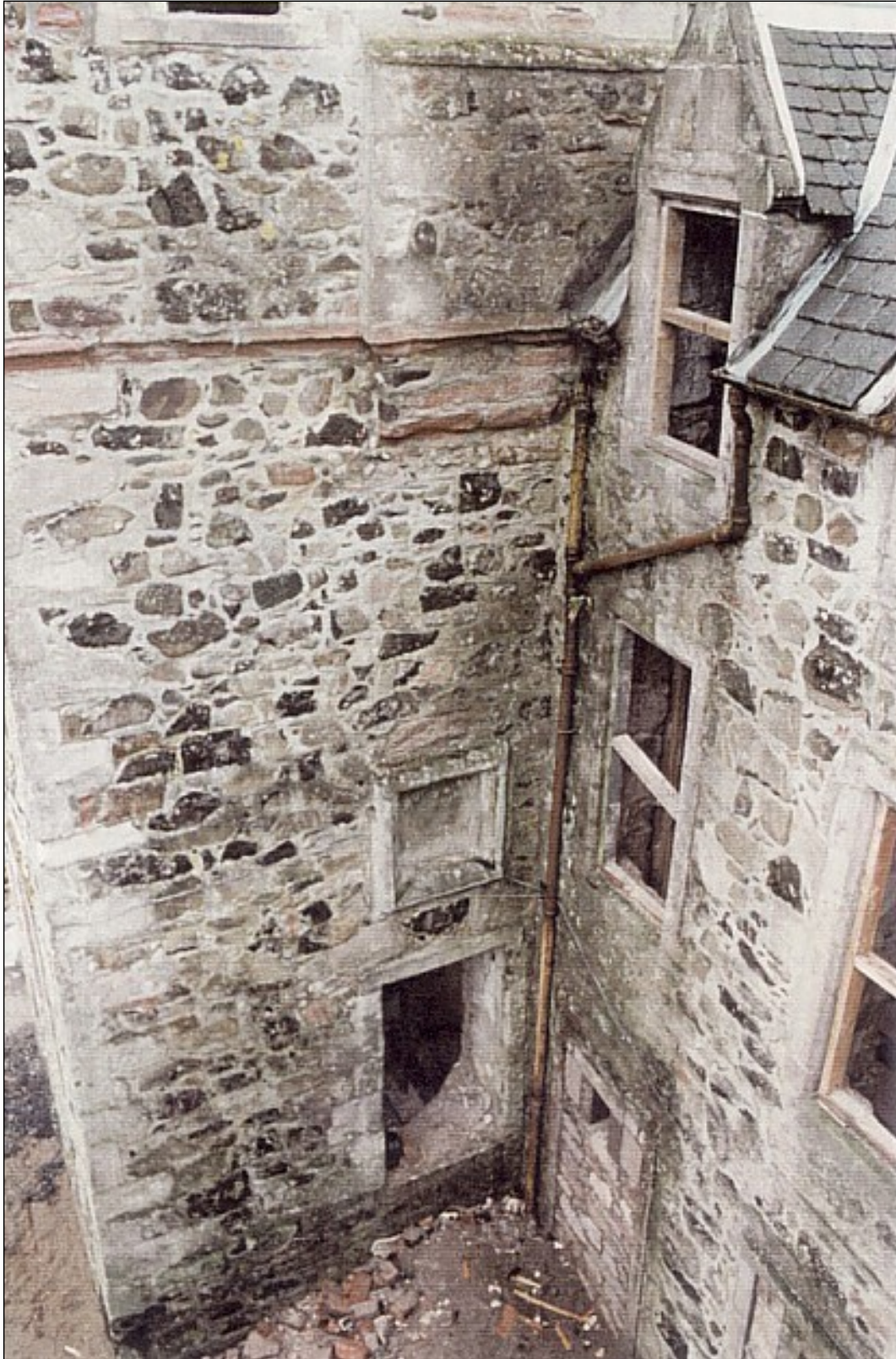
The original main entrance door in the stair turret reopened, but still stranded well above ground level.
