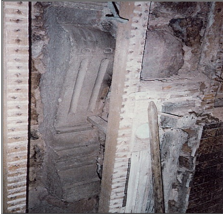
Fragment of the original great hall fireplace, found behind two later ones in the north wall.
