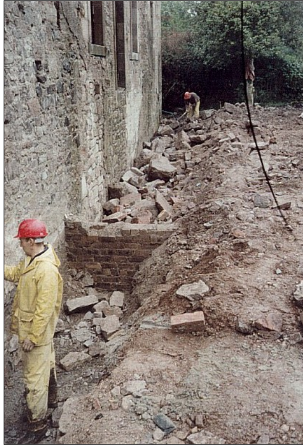
The deep trench on the west side, partly filled up. It had weakened the foundations of the west wall, but is now restored to its proper level.
