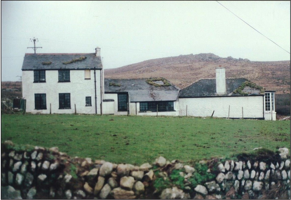
Roof damage after gales in January, 1990.
