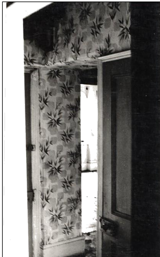
The interior of the Station Master's house had become dilapidated, but structurally the building was sound.
