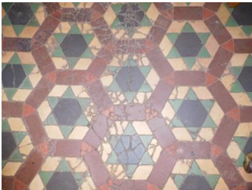
Damage had become severe in areas of heavy traffic.
