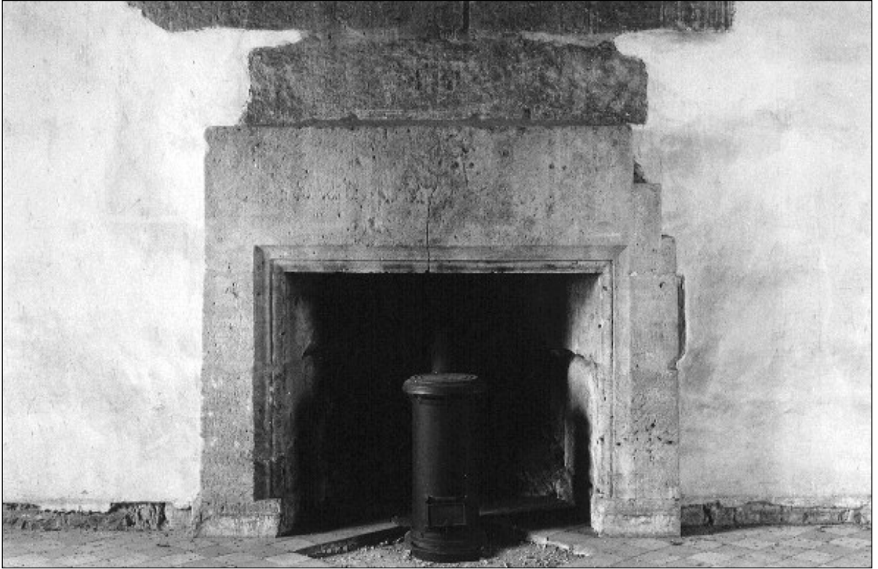
The fireplace lintel had cracked right through
