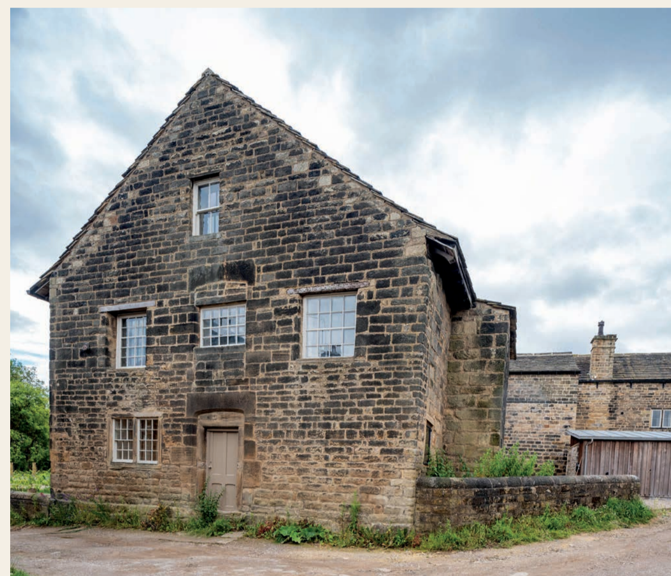
The central window on the gable of the Great Hall, once perhaps used to take in bales of wool or other goods.
